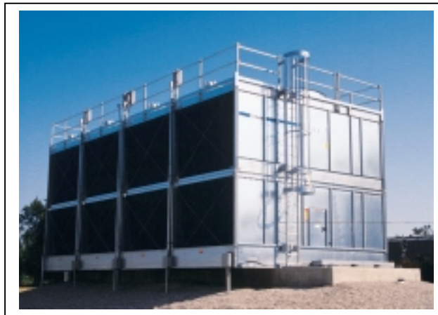
Figure 15 - Induced Draft Cooling Tower
