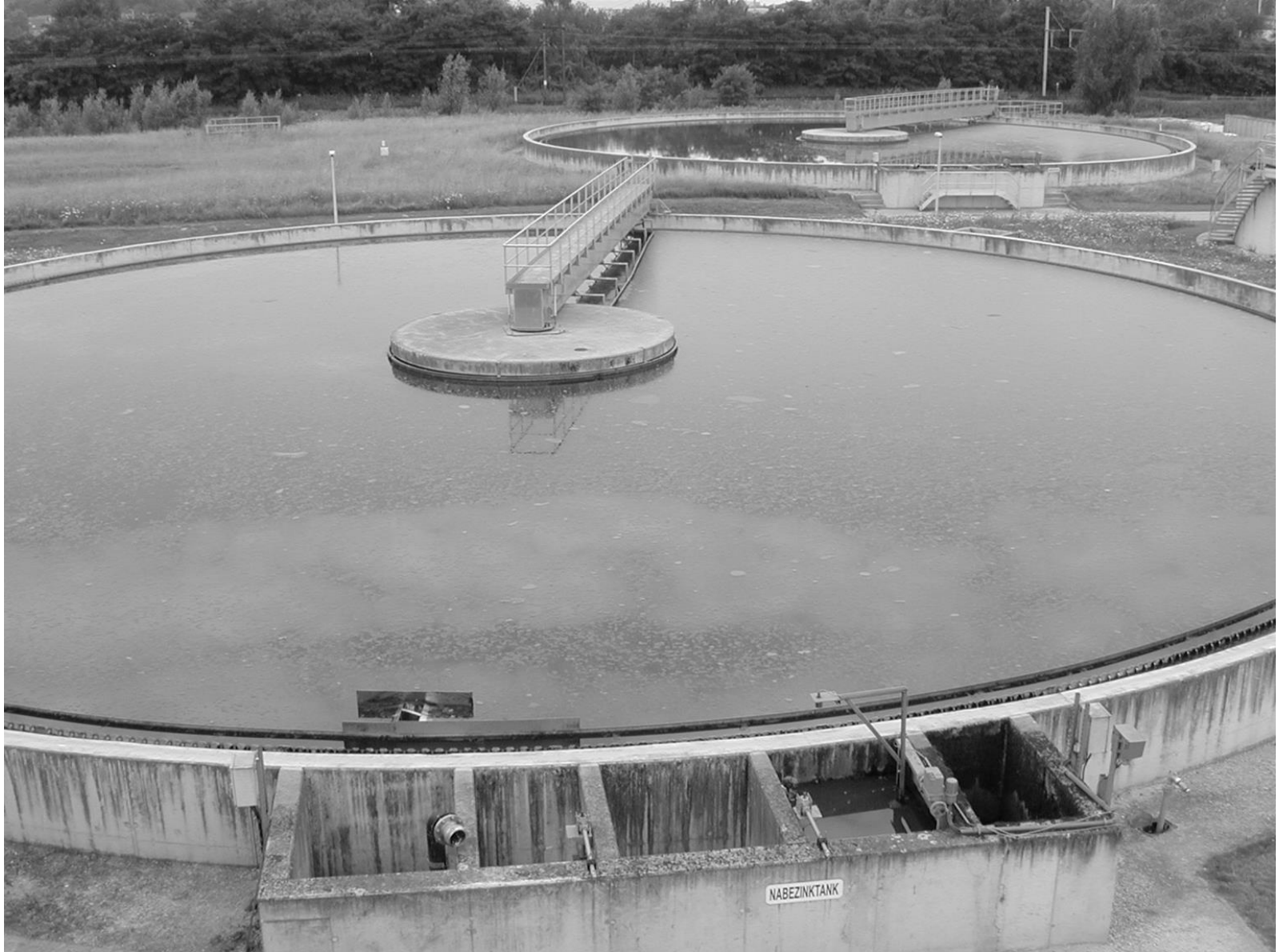
Clarifier for activated sludge process
