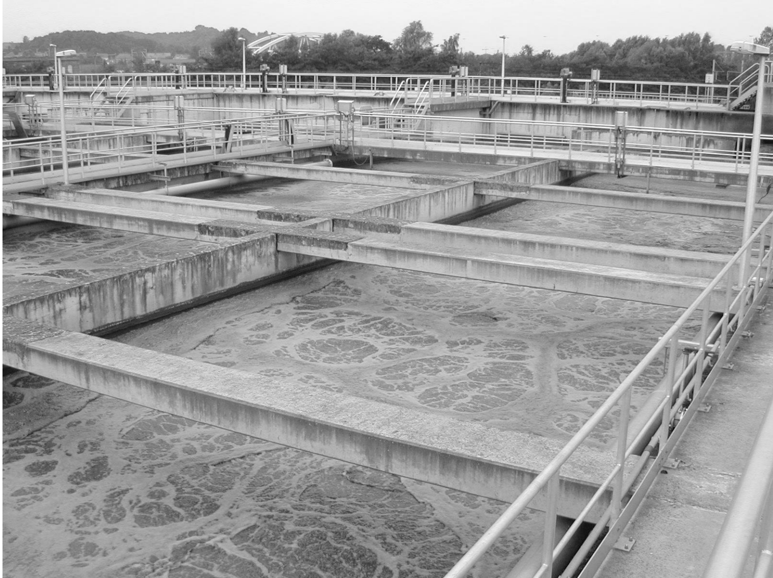
Aeration basin for activated sludge process
