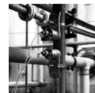
Installation in highly corrosive environment
