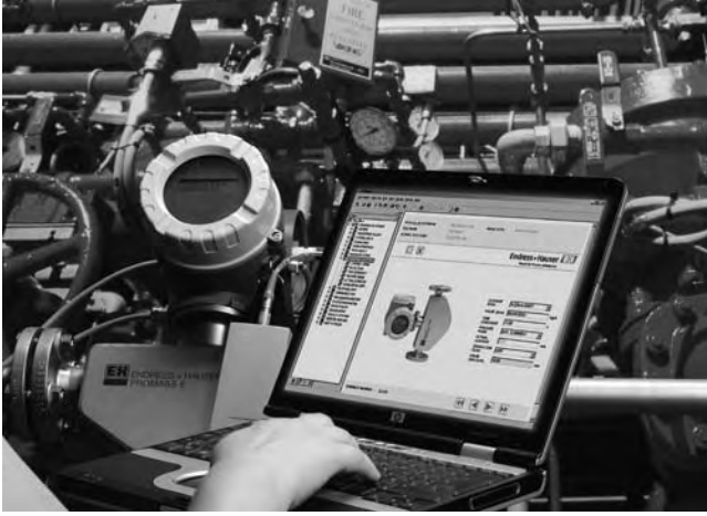
Functional check of a flowmeter using the FieldCare software associated with the FieldCheck tool (small right picture)
