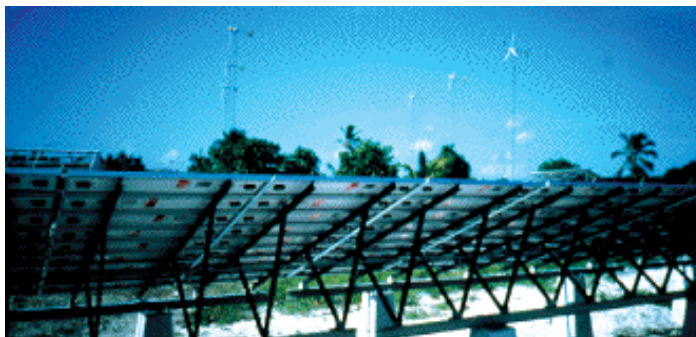
Fig. 14. Xcalak, Mexico wind turbines and PV array (1993).
