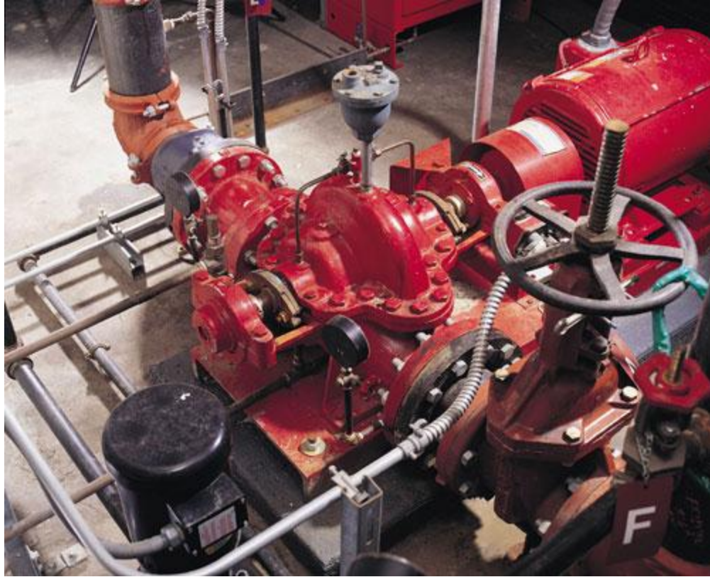
fig-3. electric pump
