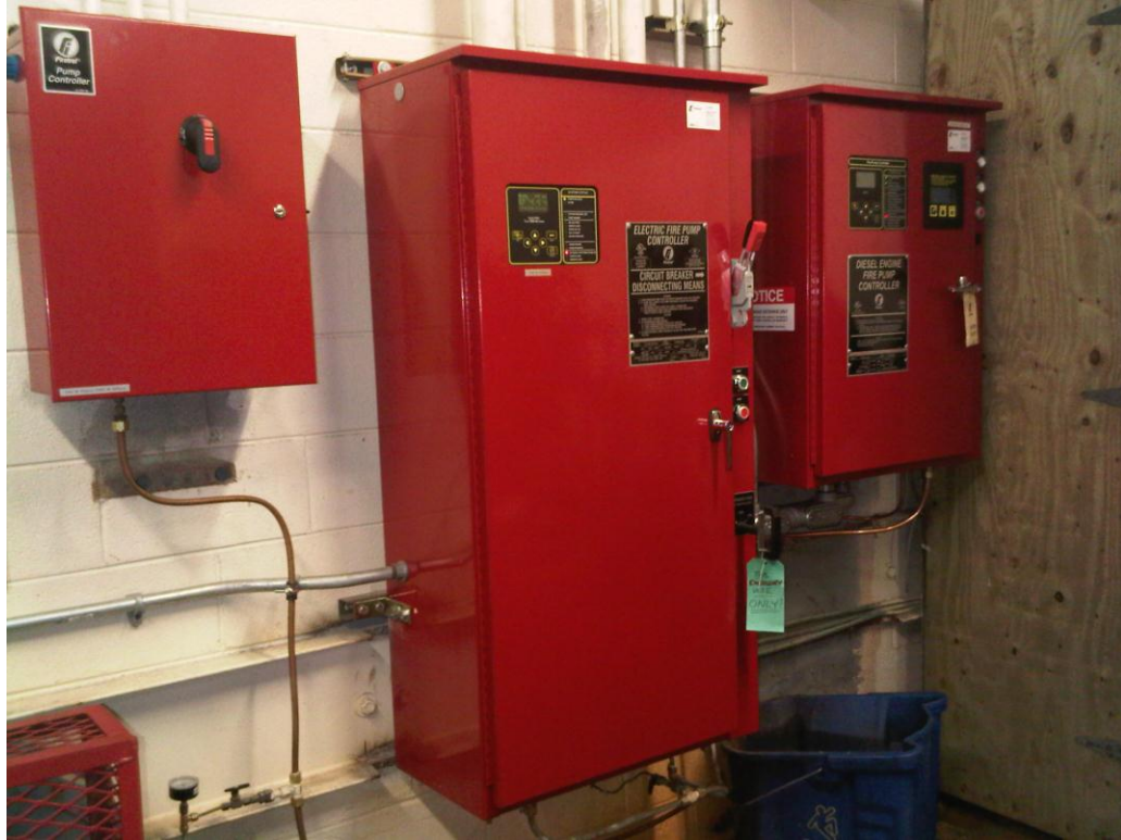
fig-5. fire pumps controllers
