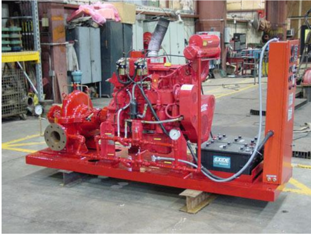
fig-2. diesel pump
