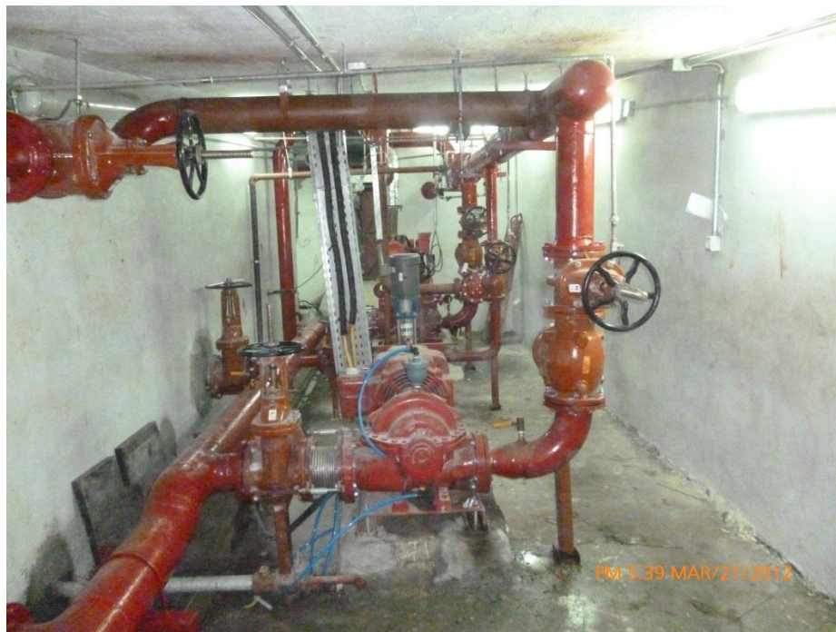
fig-8. firefighting pump room
