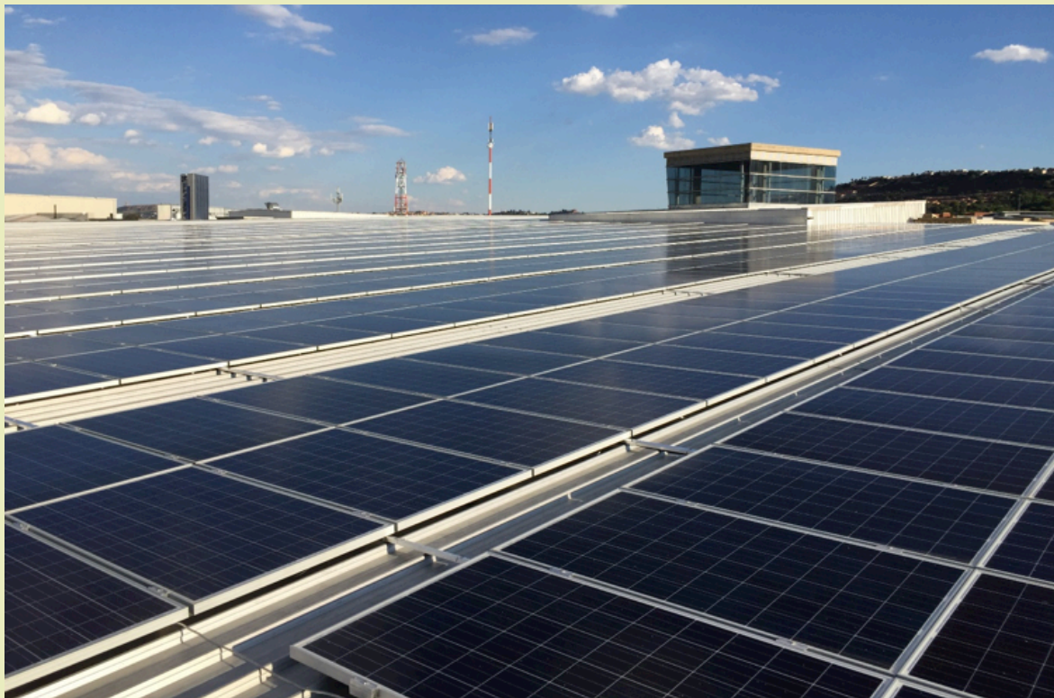
Figure 24: Clearwater Mall PV arrays
