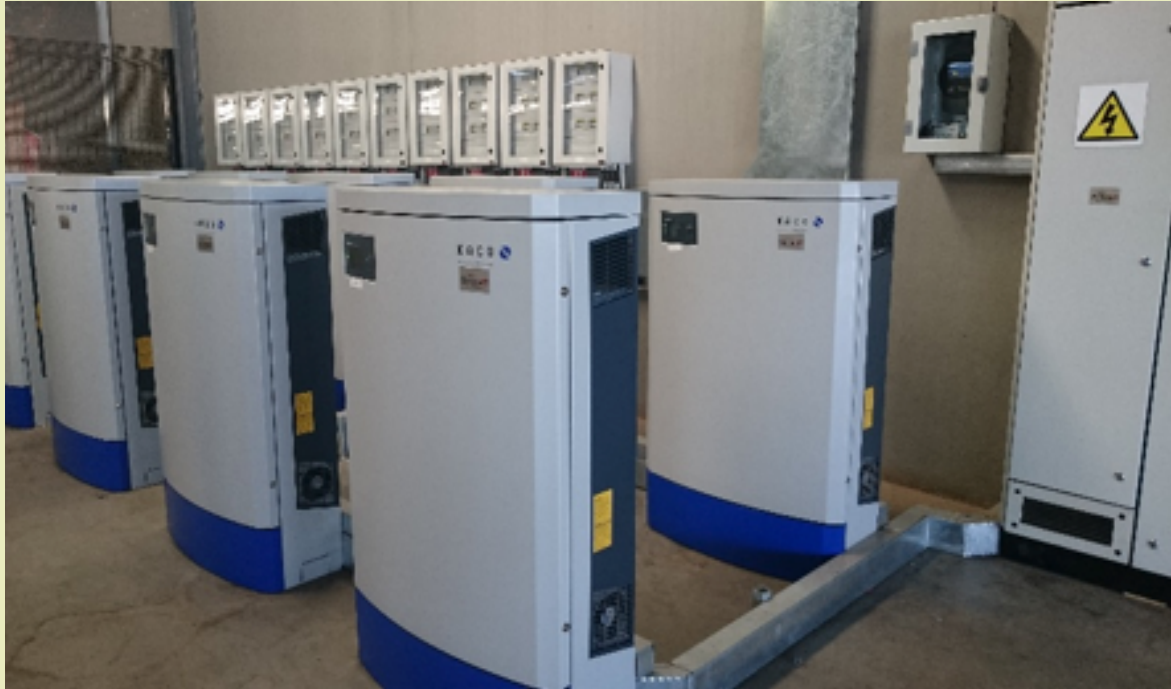
Figure 23: Clearwater Mall PV system inverter bank
