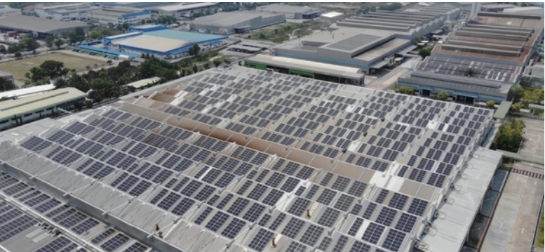
Solar panels introduced at STM
