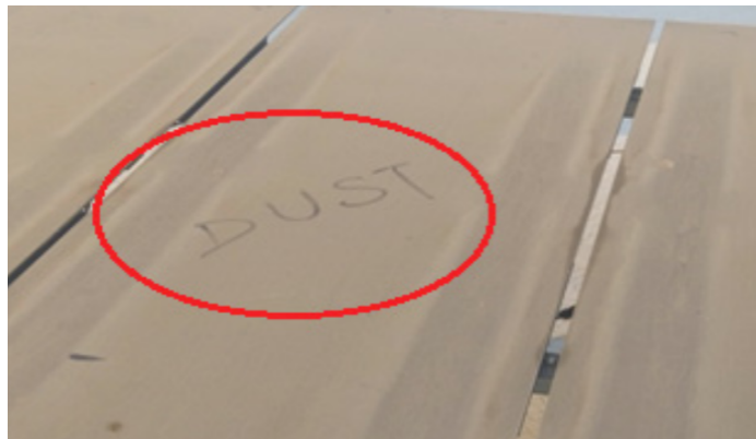
Figure 7: Dust accumulation on a solar panel
