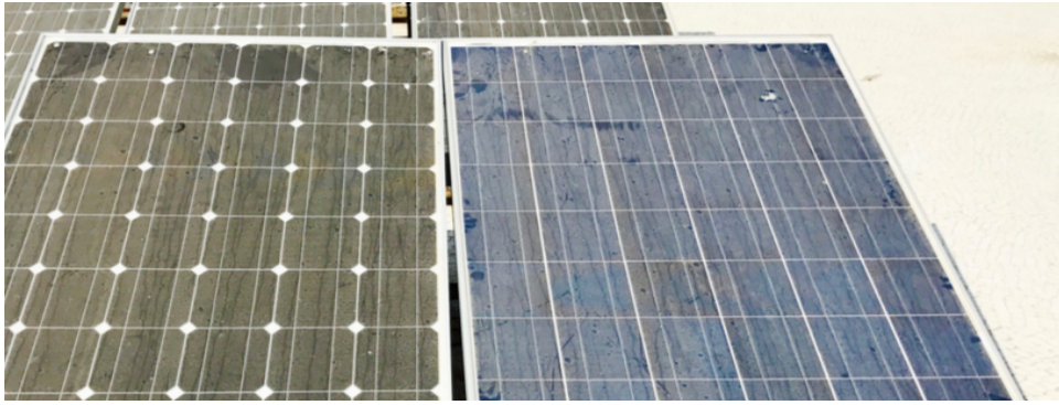
Figure 13: Different types of panels in the same installation
