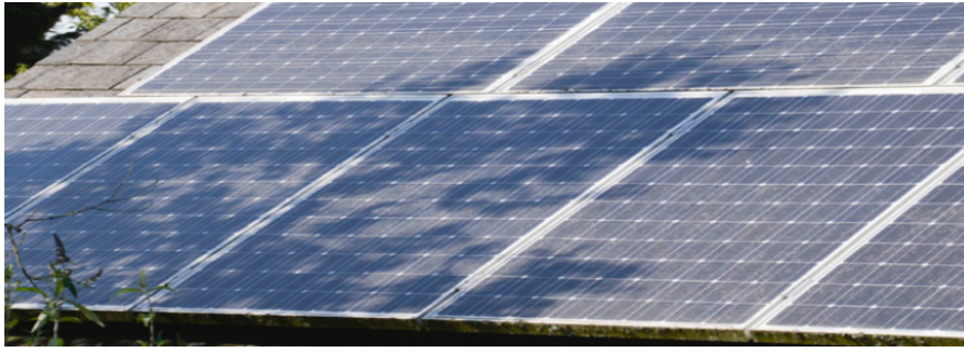
Figure 8: Shaded solar panels
