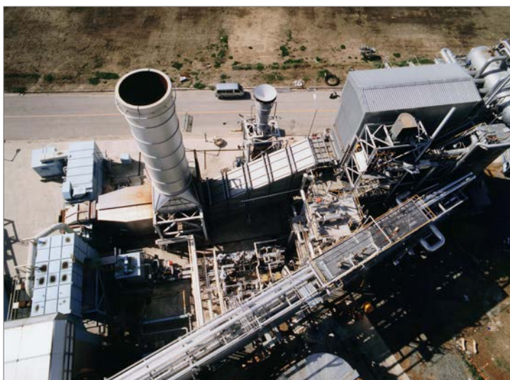
Figure 13: High hydrogen fueled 6B.03 gas turbine.
