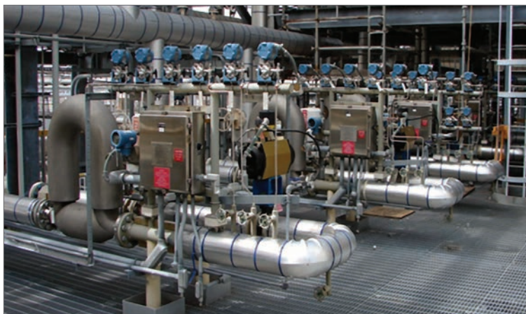
Figure 11: Hydrogen / natural gas blending system.
