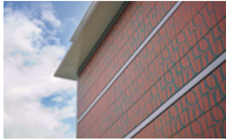
Building-integrated PV Transparent PV Design feature Coloured PV
