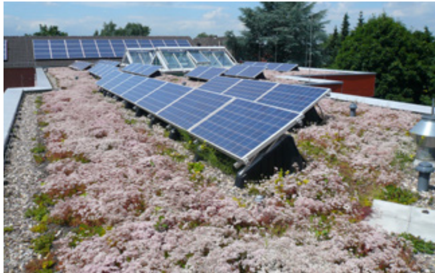
Intensive green roof & PV
