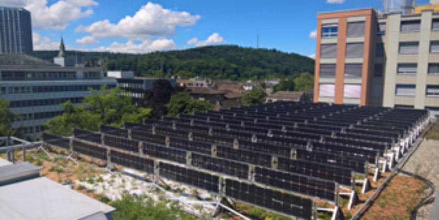
Figure 72: Rooftop experimental facility
