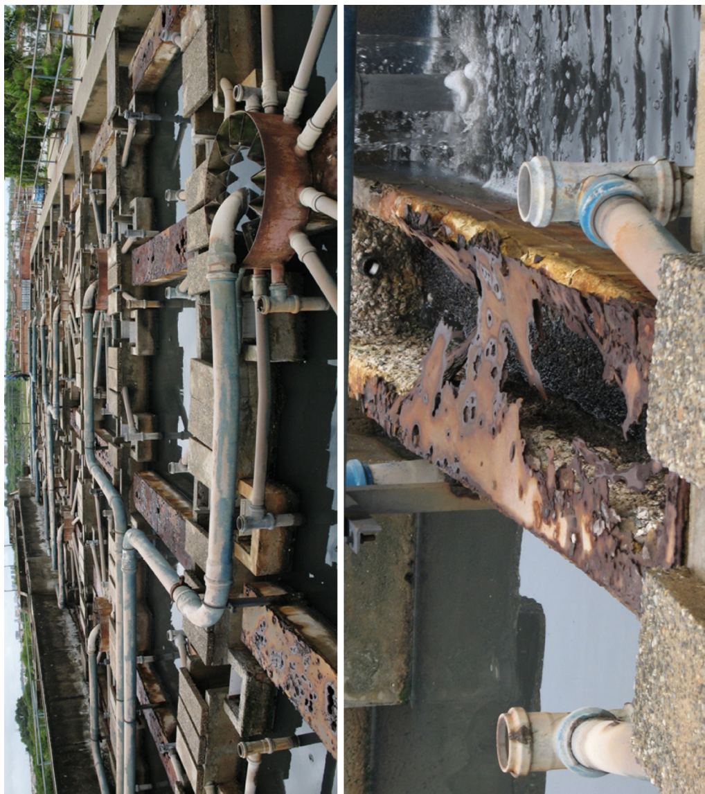
Figure 2.14 Serious corrosion problems can arise with the production of \text{H}_2\text{S} and \text{H}_2\text{SO}_4 in UASBs as shown in this unit in Aracaju, Brazil. Raw wastewater monitoring for sulfate concentrations, and the use of corrosion-resistant materials throughout the UASB, must be specified by design engineers to avoid these problems.
