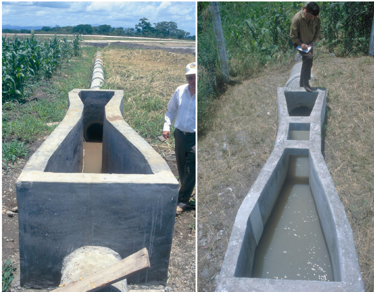
Figure 4.13 Examples of Parshall flumes that never should have been built. The dimensions are wrong, the construction is poor, and there is no headloss through the structure. For these reasons, pre-fabricated Parshall flumes that have certified calibration should always be used (left photo: Catacamas, Honduras; right photo: Villanueva, Honduras).
