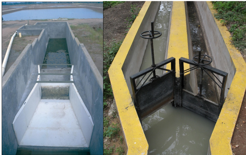
Figure 9.9 Left: A properly installed, prefabricated Parshall flume used to measure influent flowrates to a facultative pond. Accurate flow measurement is essential for assessment of hydraulic and organic loadings to the pond system. Right: Well-designed and installed sluice gates in a dual channel grit chamber; the gates have metal-to-metal contact that are routinely greased for ease of operation (left photo: El Paraíso, Honduras; right photo: Suchitoto, El Salvador).
