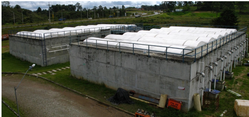
Figure 2.13 A well-designed and constructed UASB system for a population of 125,000. The methane is flared and not used as an alternative energy source (Rionegro, Colombia).
