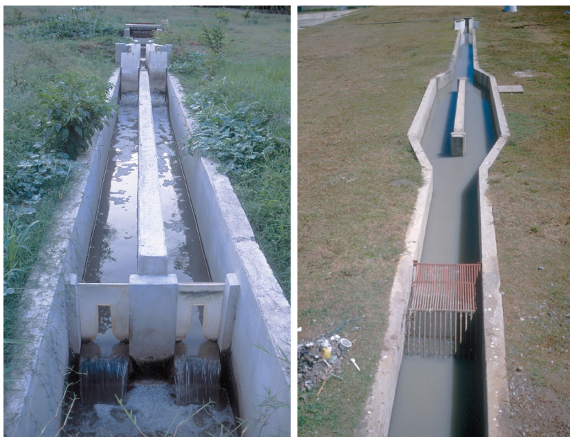
Figure 10.2 In many facilities that have grit chambers, the operators do not operate them correctly. Part of the problem is poor design and poor construction, where the grit channels cannot be sealed or drained, and part is a problem of operator training in the correct operational procedure. In the photo to the left (Trinidad, Honduras), the operator left both channels in operation for lack of a way to close them with a sluice gate. In the photo on the right (Granada, Nicaragua), there were no sluice gates to close the channels, nor a way to drain a closed channel to remove the grit.
