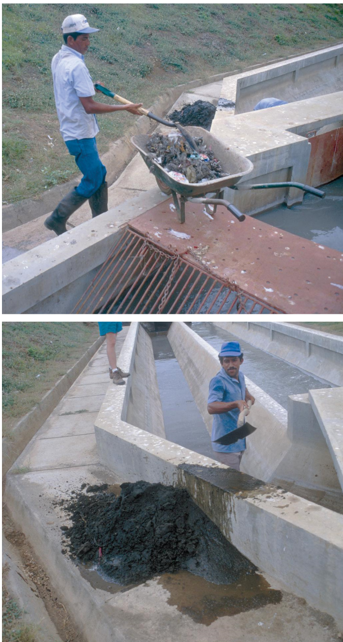
Figure 10.1 In preliminary treatment, the operator's responsibility is to clean the bar screen daily, and the grit chamber when needed – typically once a week in small systems. It is essential to agitate the settled solids in operating grit chamber on a daily basis so that entrapped organic solids escape to the downstream pond, and inorganic solids remain in the channel. The solids from the bar screen and grit chamber should be buried and covered on a daily basis (Leon, Nicaragua).
