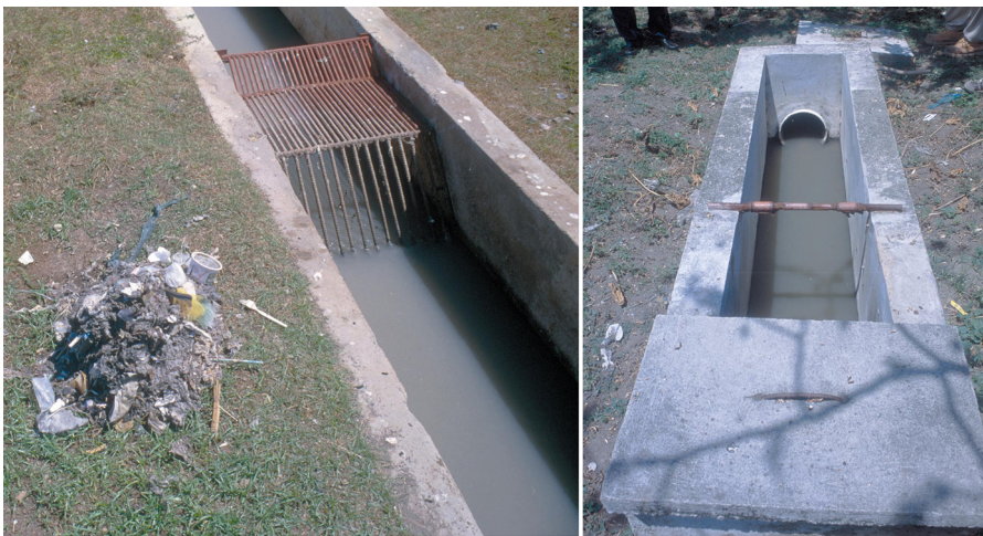
Figure 4.7 The bar screen on the left, while having an appropriate opening to retain the coarser solids and allow human feces to pass, and also a suitable drainage platform, should not be constructed of rebar. Reinforcing bars are not corrosion resistant and deteriorate rapidly in a wastewater environment where corrosion conditions are favored as shown in the right photo. The screening solids in the left photo should be buried as soon as possible to protect public health (Left: Granada, Nicaragua; Right: Choloma, Honduras).
