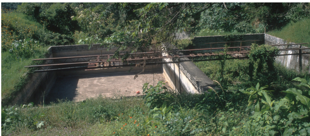
Figure 2.8 An abandoned activated sludge treatment plant in an urbanization within the city of San Salvador, El Salvador. New developments often require wastewater treatment to be approved, and activated sludge is chosen to save land area for more housing. The cost of operation and need for skilled personnel, however, is normally beyond the resources of the urbanization, and treatment plants like this one quickly fail, if they were ever in operation to begin with.
