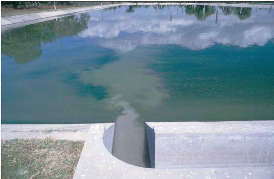
Figure 9.12 A good example of an inlet structure with open channel that enters this facultative pond at the water level. The raw wastewater plume entering the pond is clearly seen to be approximating plug flow (Granada, Nicaragua).
