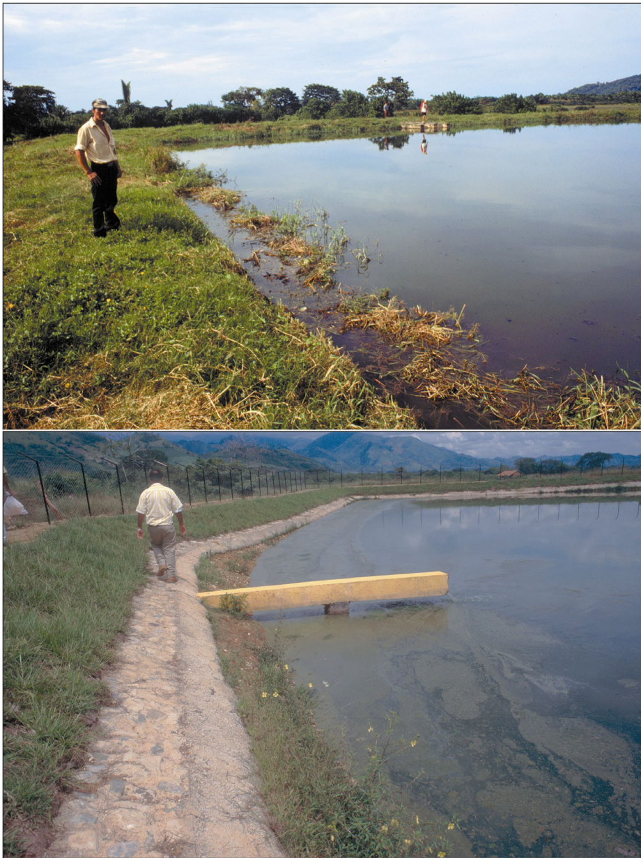
Figure 9.26 In the photo above (Tela, Honduras), the facultative pond has serious problems with the growth of aquatic plants at the shoreline due to lack of a revetment. In the photo below (Catacamas, Honduras), the poor construction of the revetment (note the contour lines at the water level) with insufficient freeboard does not prevent the growth of aquatic plants.
