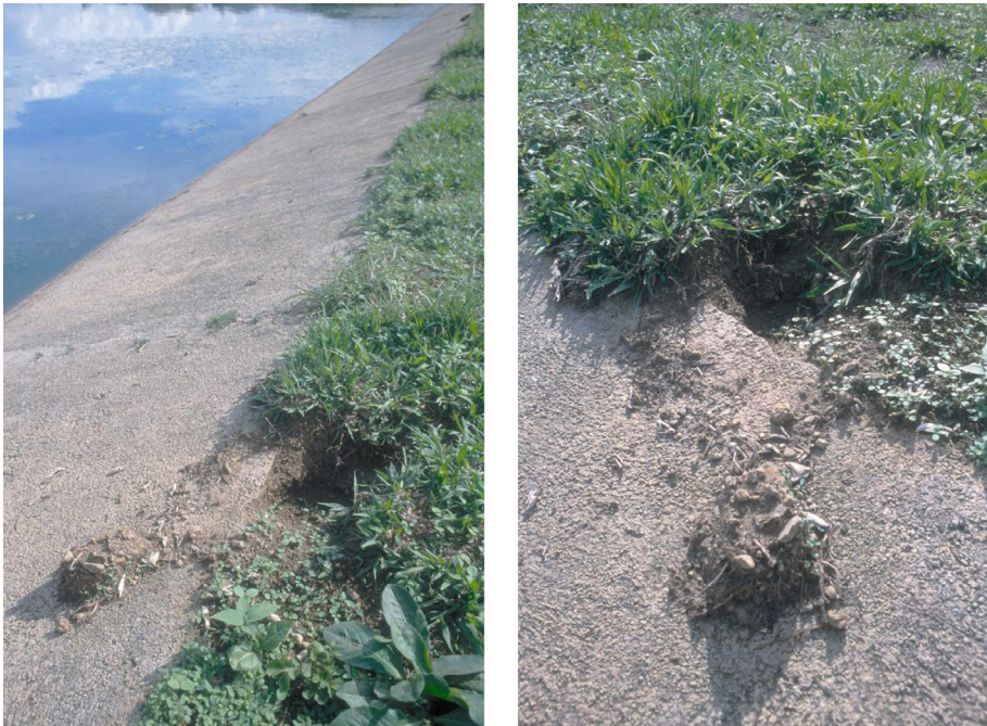
Figure 10.11 Turtle excavations behind the revetment in a secondary facultative pond. Turtles can burrow behind and under geomembrane liners and the revetment to deposit their eggs. The operator should monitor the condition of a liner and revetment routinely when there are high turtle populations in the ponds (Danlí, Honduras).
