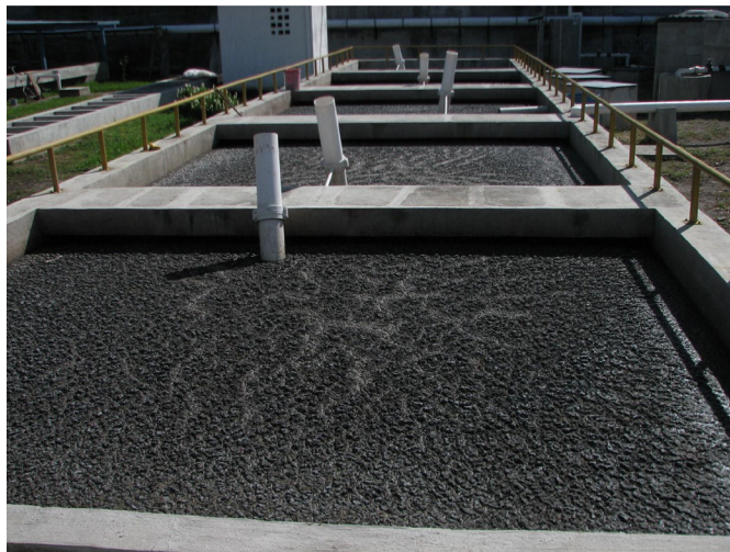
Figure 3.6 A secondary clarifier in an activated sludge treatment plant filled with activated sludge from the aeration basin that was washed out due to excessive inflow into the collection system from Hurricane Stan (Panajachel, Guatemala). The plant had no bypass channel and no pump to return the sludge to the aeration basin after the storm event; as a result, it was discharged to the anaerobic digester. Re-startup of aeration basins with raw wastewater can take many days to several weeks if there is no source of activated sludge from a nearby plant, which was the case here as this plant was the only one in the country. This problem is unlikely to happen in waste stabilization ponds with their large volumes and long retention times of weeks rather than 6 h in activated sludge plants.
