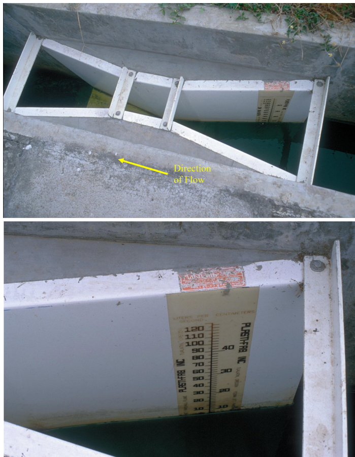
Figure 4.11 An example of a pre-fabricated Parshall flume installed for a horizontal flow grit chamber. The designer should always specify pre-fabricated and calibrated Parshall flumes in the design to avoid the construction problems shown in Figures 4.13 and 4.14 (Masaya, Nicaragua).
