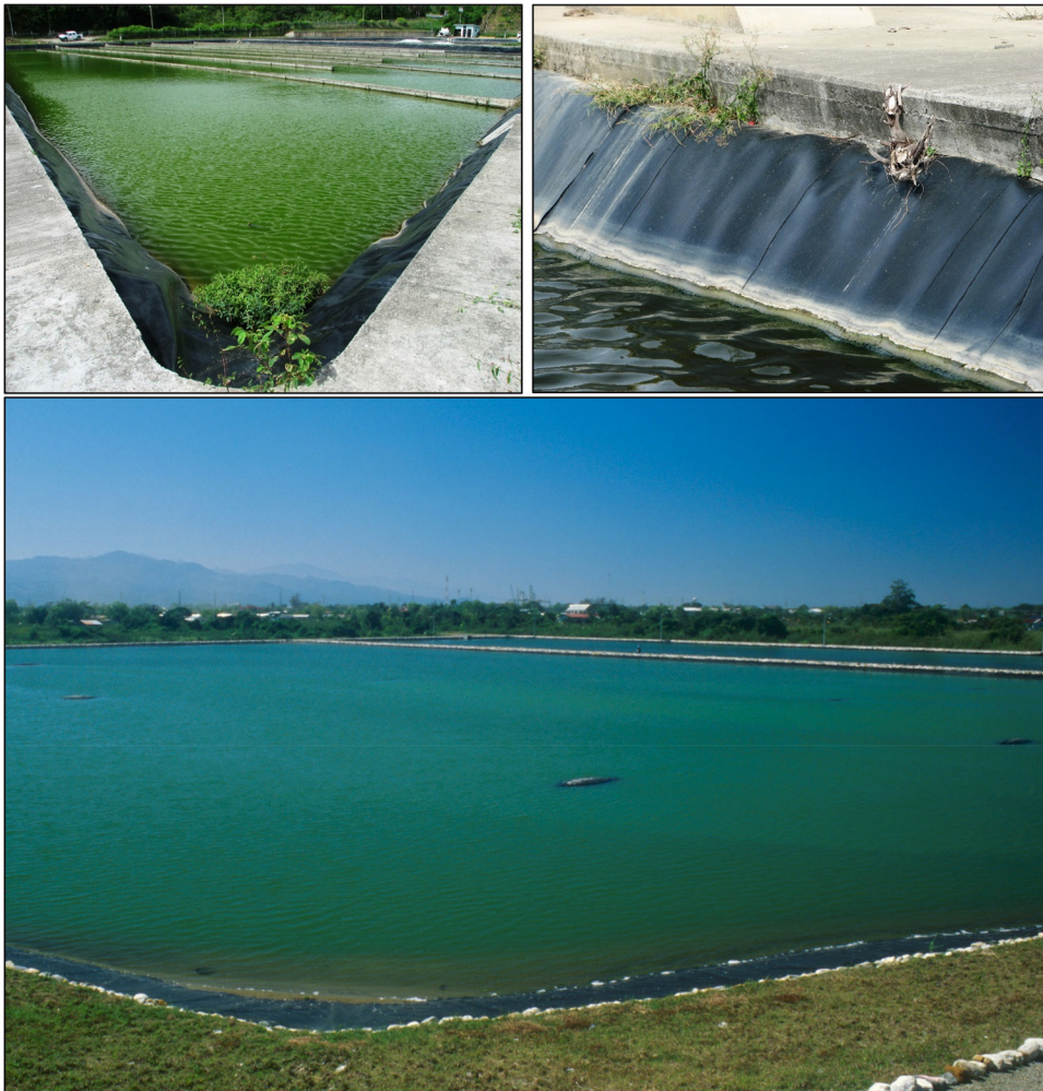
Figure 9.6 Problems encountered with geomembrane liners. In the top photos, emergent plants that were not controlled grew through the seams and tore the membrane liner at, and above, the waterline. In the bottom photo, the secondary facultative pond was built above a shallow water table influenced by tidal action. As the water table rose and fell, it formed bubbles in the membrane bottom that rose to the surface in a pond with a 1.5 m water depth. Eventually the membrane could tear from the continual stress (top photos: Roatán, Honduras; bottom photo: Puerto Cortés, Honduras).
