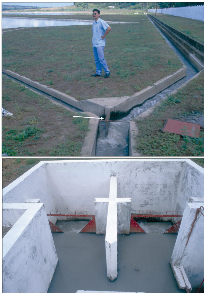
Figure 9.16 Examples of flow distribution devices between batteries of two facultative ponds in parallel. In the top photo (Masaya, Nicaragua), an adjustable partition is used (arrow). In the bottom photo (Granada, Nicaragua), a fixed partition between ponds in the center is combined with adjustable triangular weirs. The flows to each pond must be monitored to ensure equal distribution.
