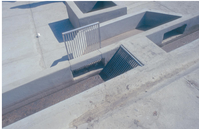
Figure 4.6 The approach channel to the bar screen should have a bypass as shown above to divert the flow during an emergency when the operator is not available to clean the screen. Note in the photo that the bars are made of aluminum. The influent bar screen should have a drainage platform as shown in Figure 4.4 (Sanarate, Guatemala).
