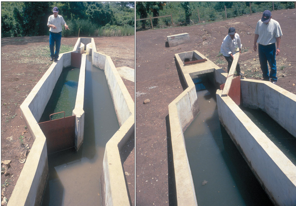
Figure 9.7 A grit chamber constructed without adequate channel drainage and well-functioning sluice gates. The channel taken out of service in the left photo was filled with stagnant water, with problems of floating scum, odors, and insects. Additionally, the sluice gate made of iron stuck tightly to the concrete track and it was supposed to slide in. The operator finally was able to pry open the sluice gate with a board, and operated both channels simultaneously – an incorrect method of operation. All grit chambers should have adequate drainage, and sluice gates that seal and slide easily (Santa Cruz de Yojoa, Honduras).
