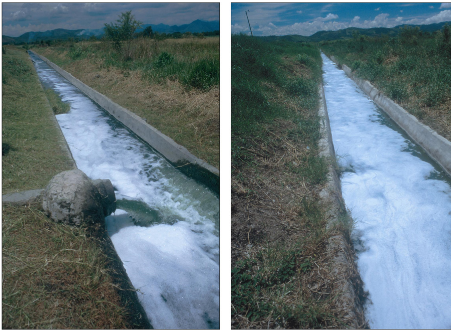
Figure 9.22 An example of the foam that can be formed by turbulence when the final discharge is above the water level in the receiving canal. Foam is caused by detergents and other non-biodegradable surfactants in wastewater. The way to control foam production is to use subsurface discharge devices as shown in Figure 9.21 (Villanueva, Honduras).
