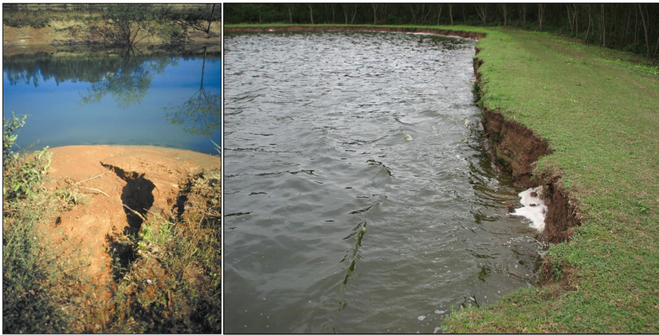
Figure 9.3 Stormwater runoff has to be controlled to protect the interior embankment slopes of ponds. Left: In this maturation pond, stormwater runoff was not controlled and caused serious erosion to the interior embankment, which did not have protection with a revetment (Zaragoza, El Salvador). Right: Wave action driven by strong winds erodes the unprotected interior embankment of this maturation pond (Santa Cruz, Bolivia).
