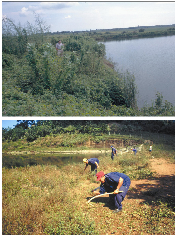
Figure 10.7 Top photo: the facultative pond has serious problems with overgrowth of weeds on the crown of the embankment down to the shoreline (note the man in the center of the photo) (Choluteca, Honduras). Bottom photo: a fundamental maintenance responsibility is the control of weed growth on pond embankments; in this photo a brigade of personnel from the National Water and Sewerage Administration (ANDA) of El Salvador cuts weeds on the embankment of a facultative pond on a supposed routine basis (Zaragoza, El Salvador).
