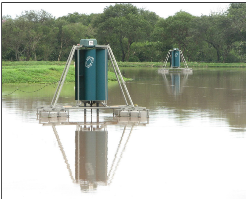
Figure 5.20 Wind-powered slow mixers in a facultative pond of the sanitation cooperative SAGAUPAC, Santa Cruz, Bolivia. If properly employed, the slow mixers greatly reduce vertical stratification and hydraulic short circuiting.
