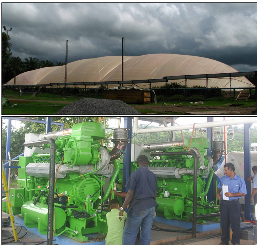
Figure 7.19 A covered anaerobic pond treating high-strength palm oil wastewater designed to capture methane for electricity generation using 750 kW gas motors. A city the size of Ouagadougou could, in theory, have a similar facility for fecal sludge treatment at the existing waste stabilization pond site, with the added benefit of electricity generation from renewable energy. Well-digested in-pond sludges would be pumped to sludge drying beds, with the leachate returned to the headworks; dewatered sludges would be stored for a minimum of 2 years to satisfy the WHO guidelines for agricultural reuse. Monitoring would be necessary to ensure pathogen inactivation. (Agrocaribe palm oil facility, Puerto Barrios, Guatemala).
