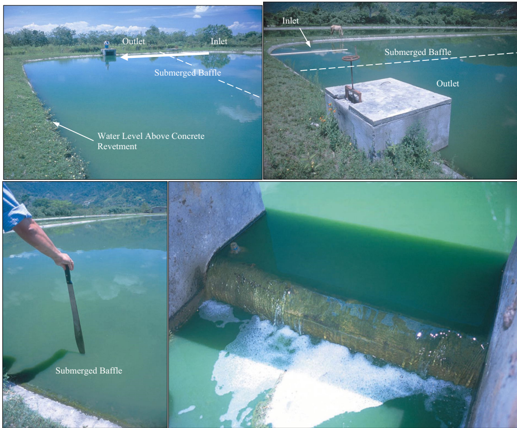
Figure 9.20 An example of poorly designed outlet devices, especially the outlet weir, in a maturation pond. The water level is above the concrete revetment, and the pond-length baffle is submerged. As a result, there is a hydraulic short circuit that allows the influent to pass directly to the outlet structure, negating the entire volume of the pond. The effluent weir is made of concrete and is not adjustable, and is located inside a concrete vault with a heavy concrete lid that could not be opened by the operator. The operator was unable to adjust the level of the pond to control the water level. Outlet structures should have adjustable sluice gates, adjustable flashboards, and open channels for operation and maintenance (Choloma, Honduras).
