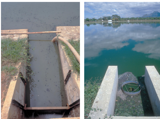
Figure 10.6 Left photo: the outlet of a facultative pond designed with a bottom sluice gate and a rectangular weir did not have the sluice gate in place; as a result, the floating solids were carried out with the effluent over the rectangular weir, and the removal efficiency of fecal coliforms was low (Catacamas, Honduras). Right photo: a circular baffle is used to control the discharge of scum in the effluent of a facultative pond (Chinendega, Nicaragua).
