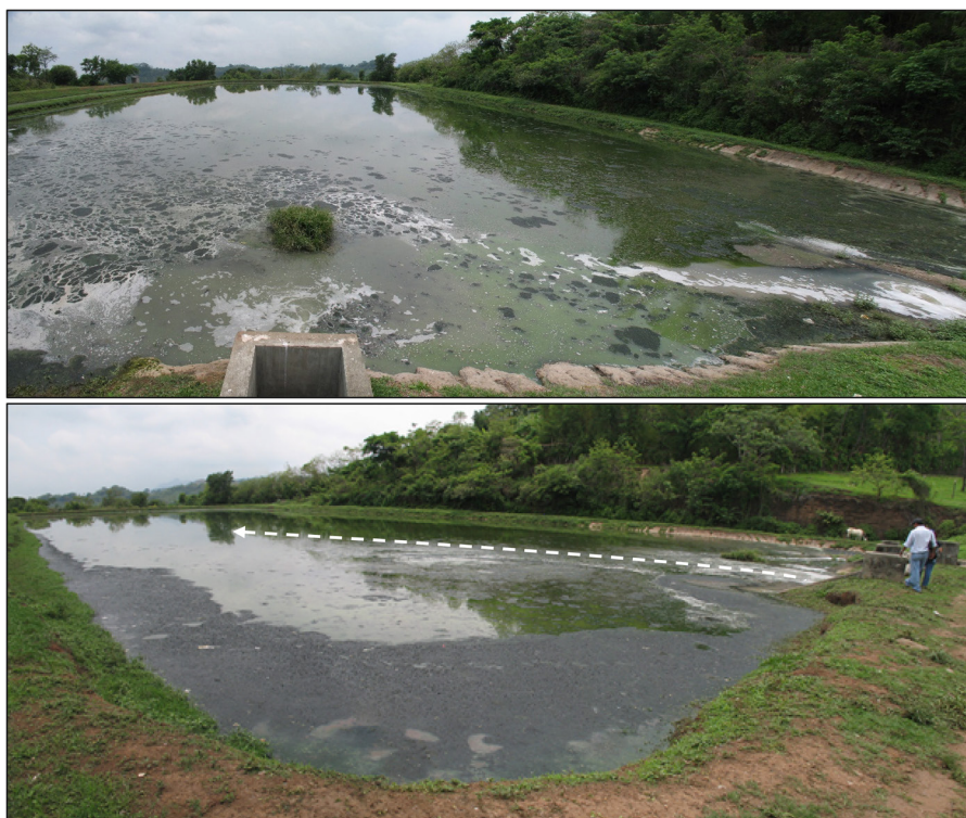
Figure 5.21 Single inlets in facultative ponds such as this one cause sludge accumulation immediately downstream of the inlet. The sludge accumulation in turn diverts inflow, forming preferential flow paths and dead zones, reducing the hydraulic efficiency of the pond (Zaragoza, El Salvador).
