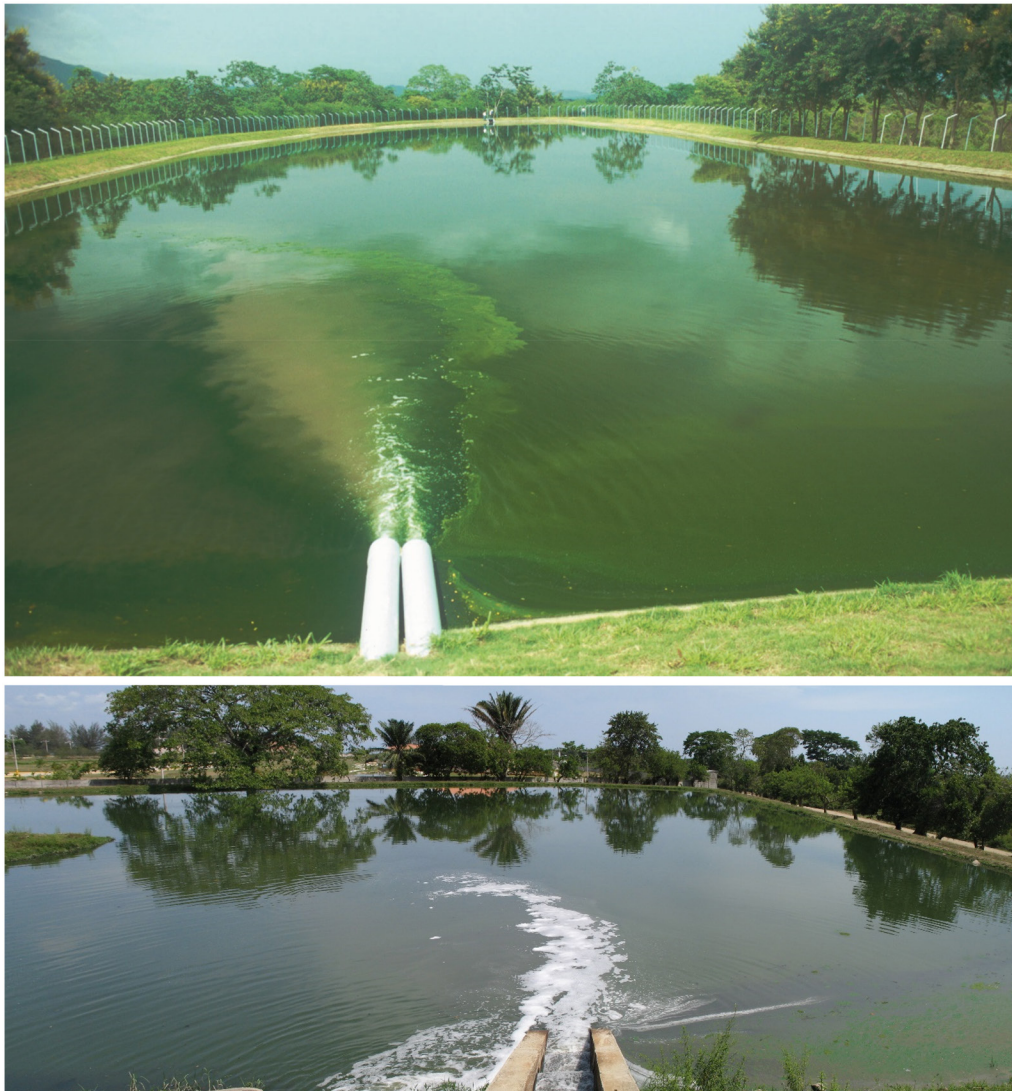
Figure 6.7 Inadequately designed unbauffed maturation ponds with significant hydraulic short circuiting. In the top photo the single inlet, discharging above the water surface, creates a 'jetting effect' (Shilton and Sweeney, 2005), where the influent jets to the left sidewall, leaving half of the pond as a dead space ( l/w = 5/1 ). The bottom photo shows a cascading influent jetting into the water surface, and drifting to the left-center, in a large, irregular pond. Note also the potential problem of shading of the water surface by trees in both ponds. (Top: Catacamas, Honduras; Bottom: Tela, Honduras).
