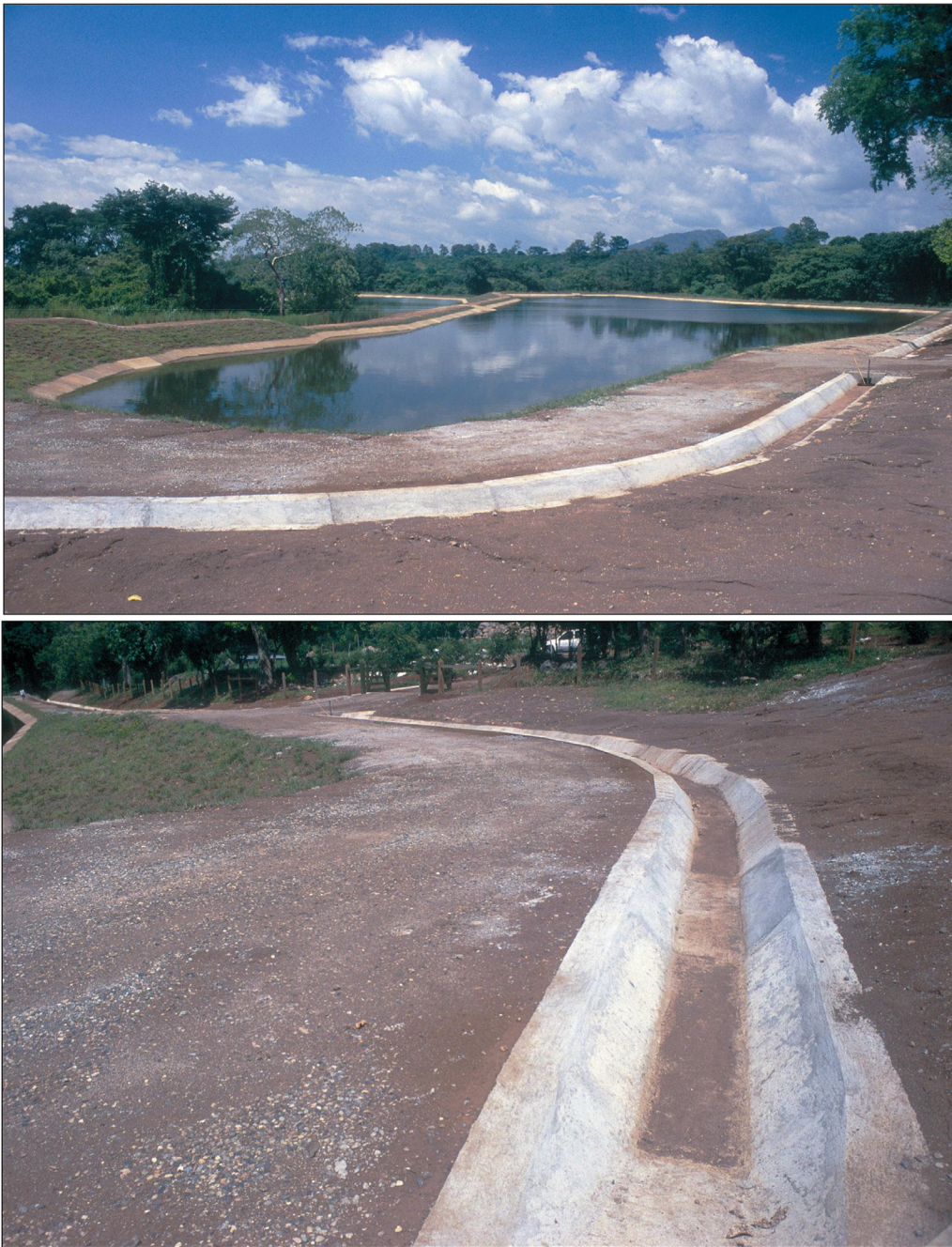
Figure 9.2 A well-designed and constructed stormwater diversion channel. If the location of the pond system is downstream of stormwater runoff, channels must be used to divert the runoff to avoid erosion of the interior embankment slopes (see Figure 9.3 ), and the input of non-wastewater suspended solids is carried by the runoff (Santa Cruz de Yojoa, Honduras).
