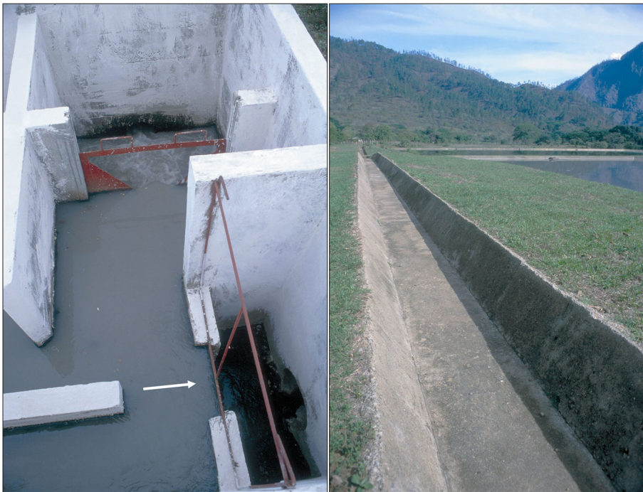
Figure 9.24 Examples of overflow weirs and bypass channels to protect a pond system from hydraulic overloads during storms. The weir on the right (arrow) in the left photo can be adjusted by the operator when required; when the water level rises above normal during storm events, the excess flow is discharged into the bypass channel. (left photo: Granada, Nicaragua; right photo: Danlí, Honduras).
