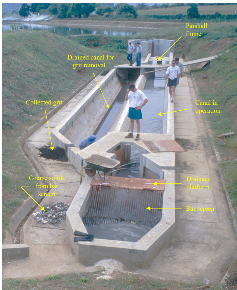
Figure 4.1 Bar screen and grit chamber, followed by a pre-fabricated Parshall flume to control horizontal velocity in the grit chamber and measure flow rates. Above the bar screen is a drainage platform to drain the screenings before removal and burial. The grit chamber has two canals: the flow is diverted to one, while the other is drained to remove solids. This grit chamber was installed because of excessive grit load to the downstream stabilization pond, which was filling prematurely with inorganic sludge. Note the piles of the screenings and the grit removed by the operator, and the wheelbarrow is used to carry the solids to their burial site (León, Nicaragua).
