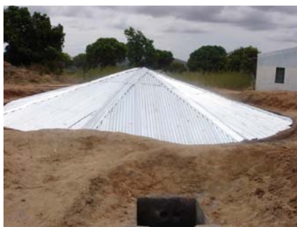
Figure 11.7 Underground tank (150,000 liters). (Source: Author's own).
