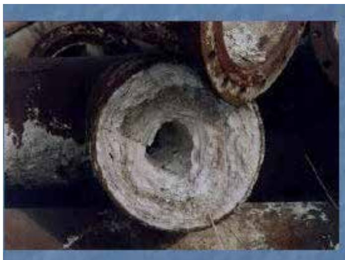
Figure 4. The build-up of scale on the interior of a pipe
