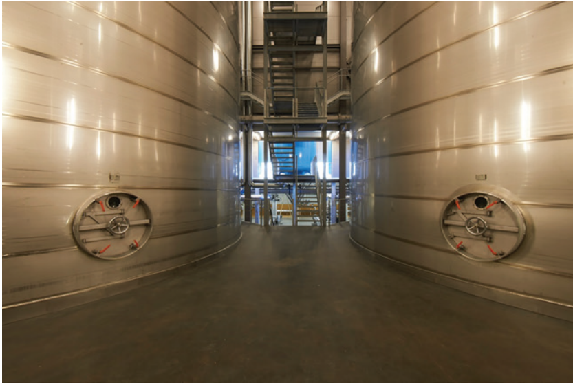
Figure 14.8 Water tanks in stainless steel that can be visually inspected.
