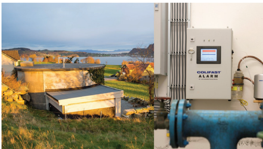
Figure 6.5 One of the first Colifast ALARM installations at a reservoir far out on the water distribution network. Mosteroy Island, Stavanger, Norway, 2010.
