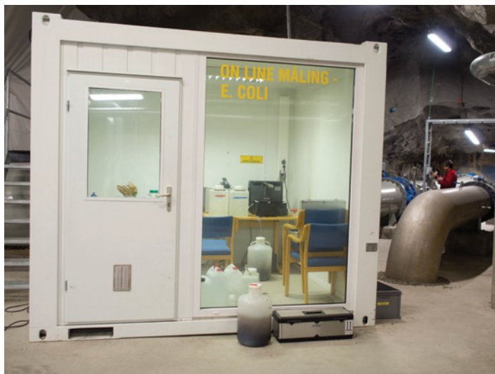
Figure 6.3 Remote CALM installation at a raw water intake. Lake Stoelsvann in Rogaland, Norway.
