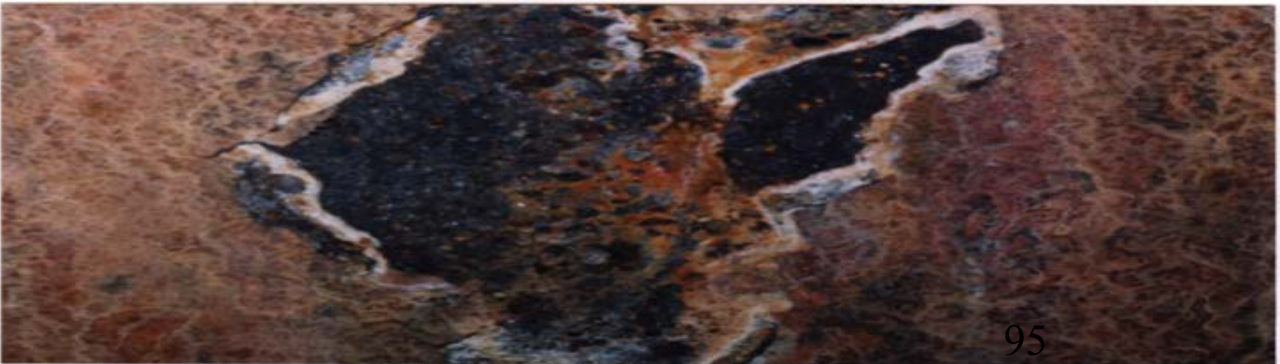
corrosion in the distillate tray
