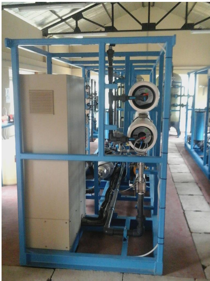
Figure 25 RO Plant- Delf Island
