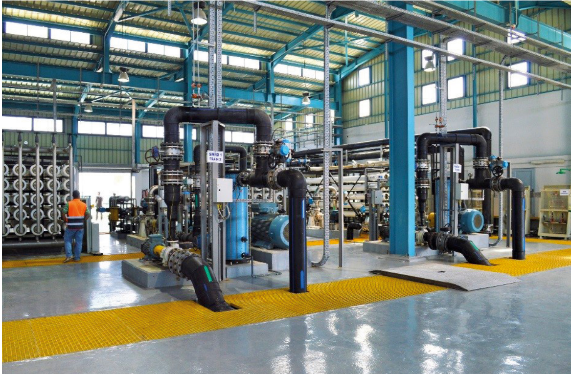
Figure 15: Khan Younis Short Term Low Volume Desalination Plant
