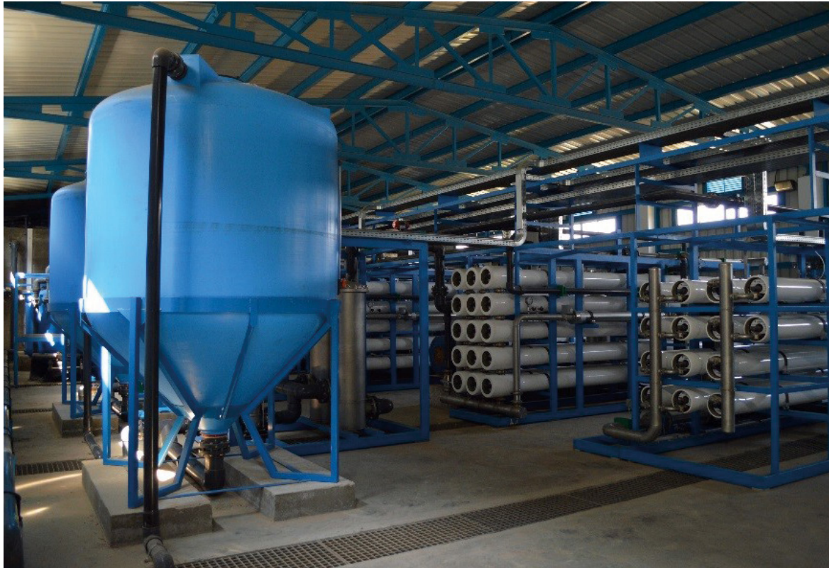
Figure 16: Deir Al Balah Short Term Low Volume Desalination Plant
