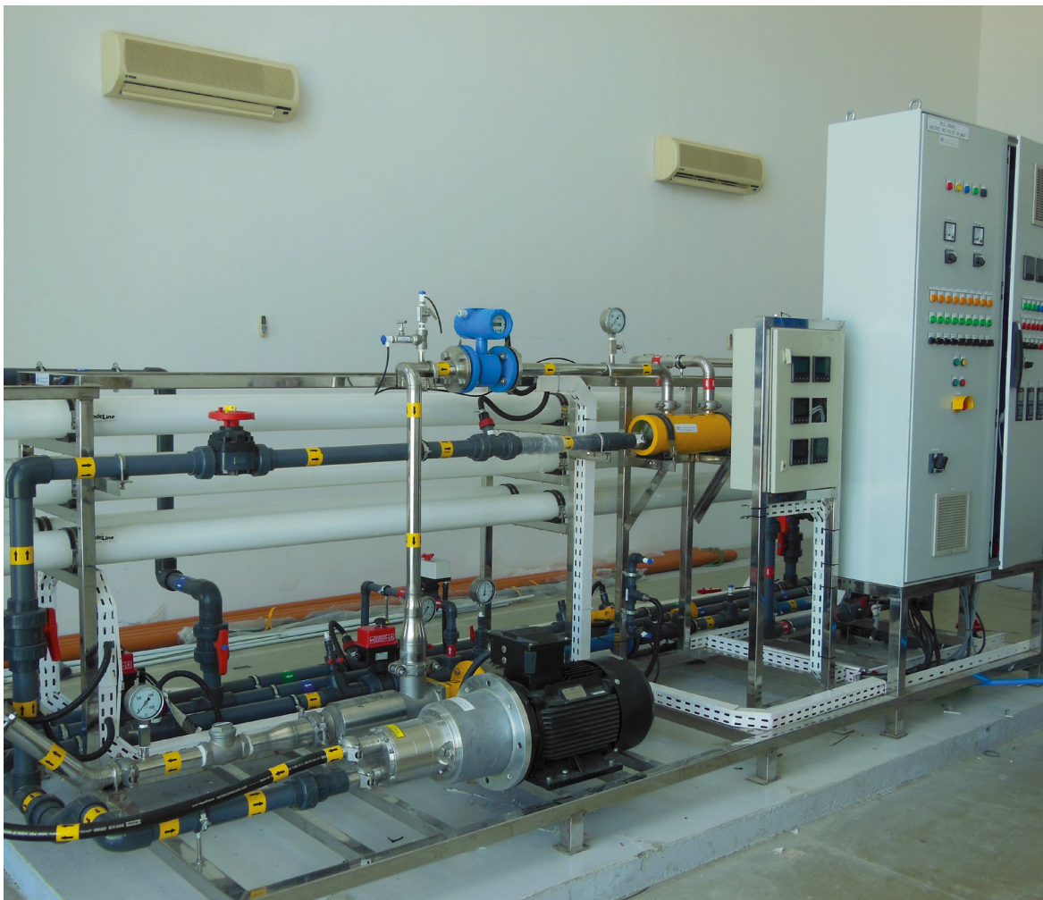
Figure 3: MEDRC RO pilot plant (RO System – 2 stages)
