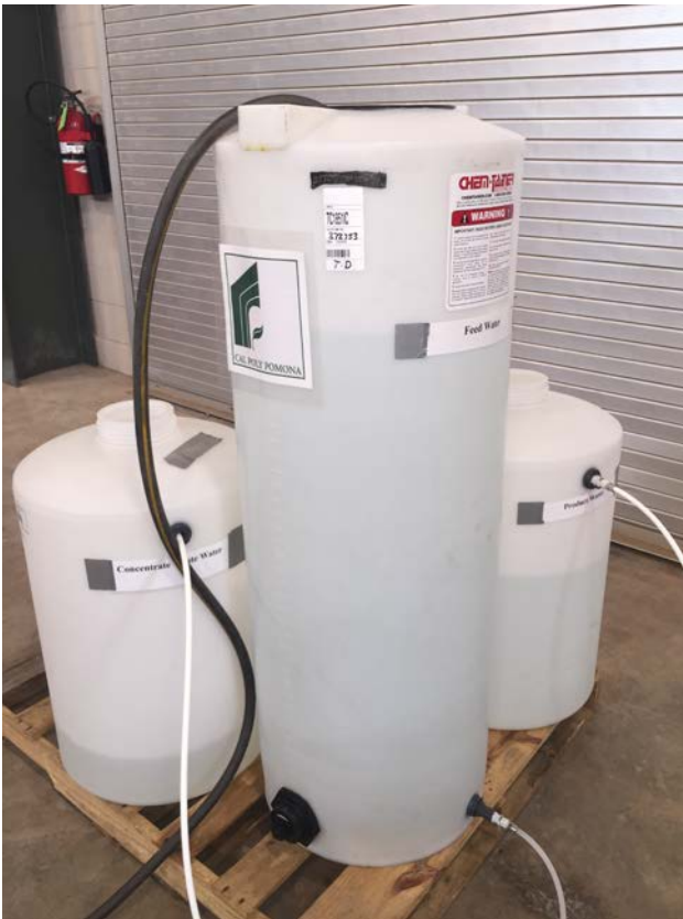
Figure 29. Feed tank, product tank, waste tank.
