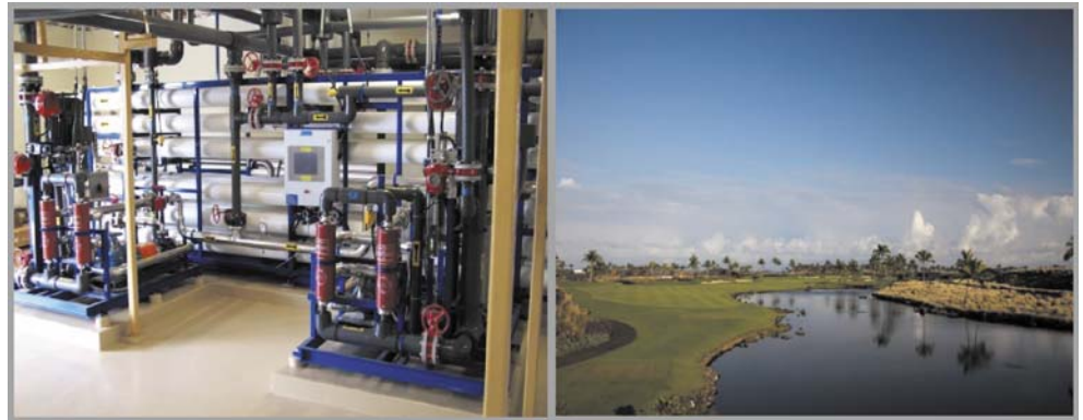
Figure 9. Brackish PX Installation
