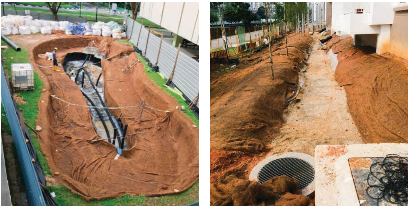
Fig. 5.6 ECM to prevent erosion and prevent silt from entering the ABC Waters design features
