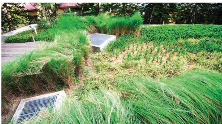
Fig. 10.38 Soak away rain garden in Anglican High School (above) and a close-up of the two separate discharge sumps (below)
