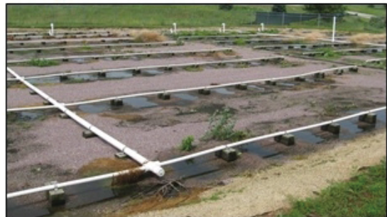
Neglected Recirculating Media Filter
