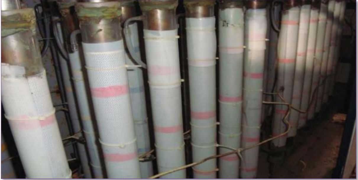
Figure 8.3: Inside View of an Ozonator (Supplied by Shivasu) installed at M/s Sri Vidya Industries, Erode
