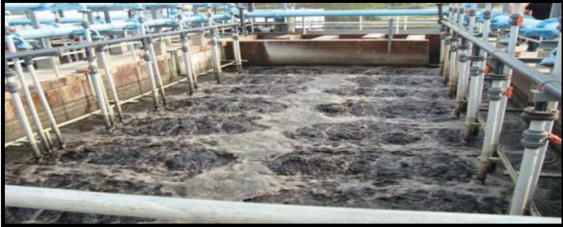
Figure 5.12 Membrane Bio Reactor installed at Angeripalayam (Tiripur, Tamilnadu) CETP
