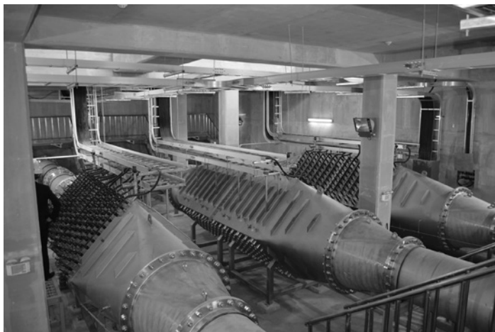
Figure 2.19 UV system installed at Siheung WTP, South Korea.
