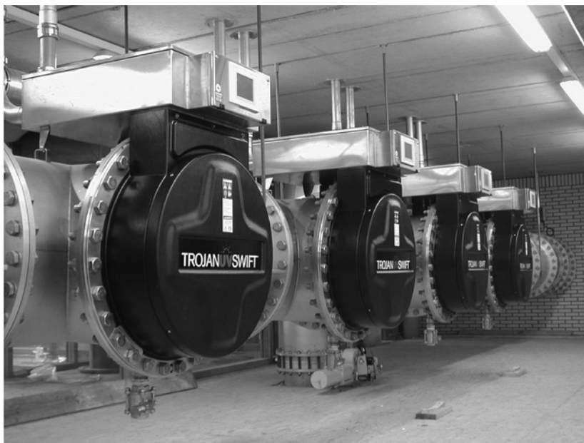
Figure 2.16 TrojanUV SwiftECT™ 16L30 reactors in Andijk III, Netherlands.
