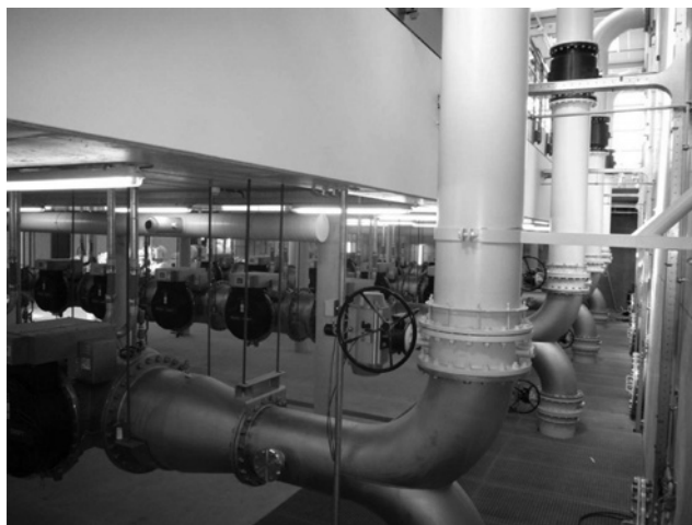
Figure 15.4 Full scale MP UV/H 2 O 2 AOP installation at PWN (6,000 m 3 /h; 0.54 kWh/m 3 ; 0–15 ppm H 2 O 2 ).
