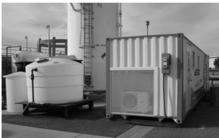
Figure 14.8 AOP Pilot setup at the Terminal Island Water Reclamation Plant.
