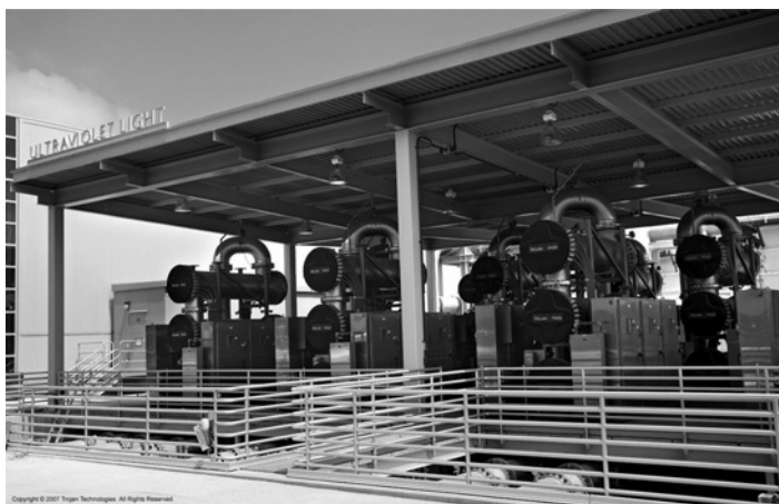
Figure 14.1 UV/H 2 O 2 AOP System at the Groundwater Replenishment System, Orange County, CA, USA.
