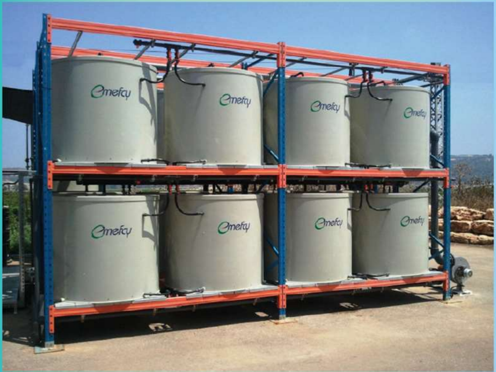
SABRE wastewater treatment plant 50 m 3 /d (13,000G/d)
