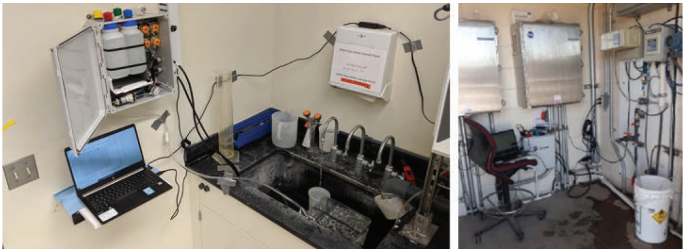
Figure 1. On-site bromide sensor installation at Nevada water treatment plant (left) and Arizona water treatment plant (right)
