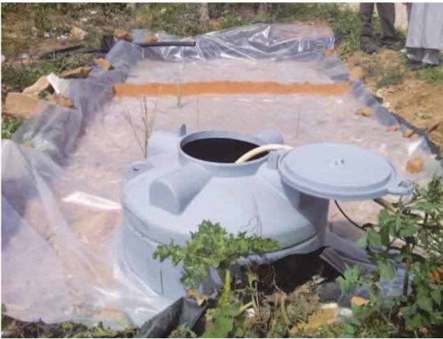
Figure 8.4: Treatment ditch at Jerash, Jordan.
