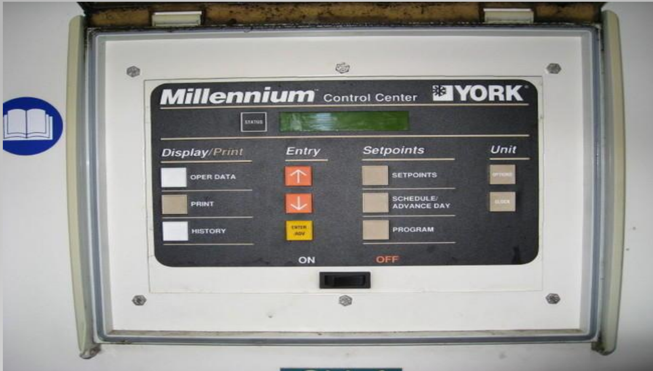
Chiller control panel
