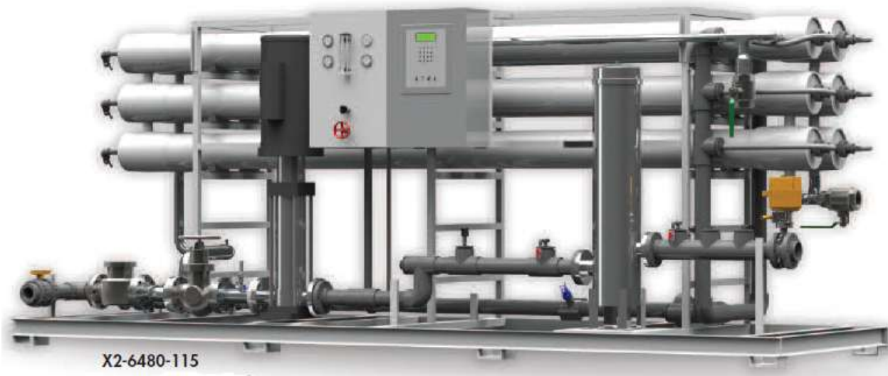
Figure 6.18 : R.O skid of Alkrameh plant
