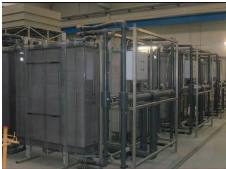
Fig. 4. EDR stacks at the Depurbaix WWTP.
