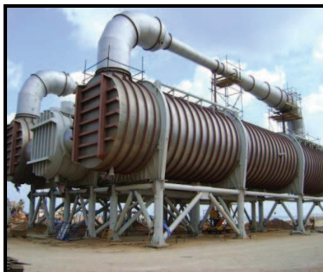
(a) Circular vessel evaporator.
