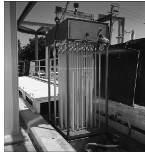
Canal disinfection equipment (Mostly in wastewater disinfection)
