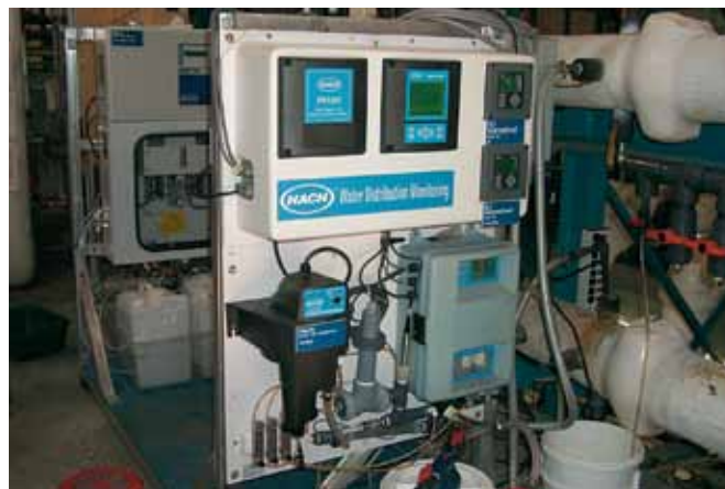
Figure 2.7 DSS Loop No. 6 - Online Instrumentation
