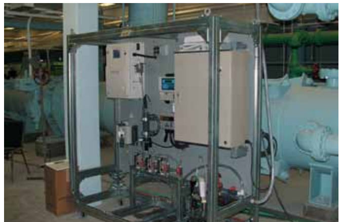
Figure 2.13 First Pilot Utility - Water Security Initiative Instrument Panel Type B
