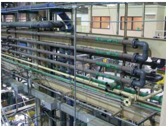
Figure 2.5 Single Pass DSS – Connecting Pipe Elbows
