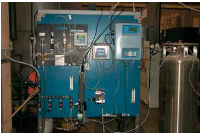
Figure 3.1 Single Pass DSS Instrument Panel at 80-foot Sampling Location
