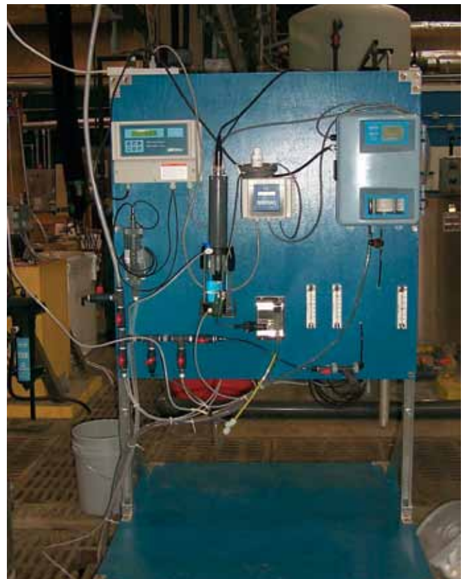
Figure 3.2 Single Pass DSS Instrument Panel at 1,180-foot Sampling Location
