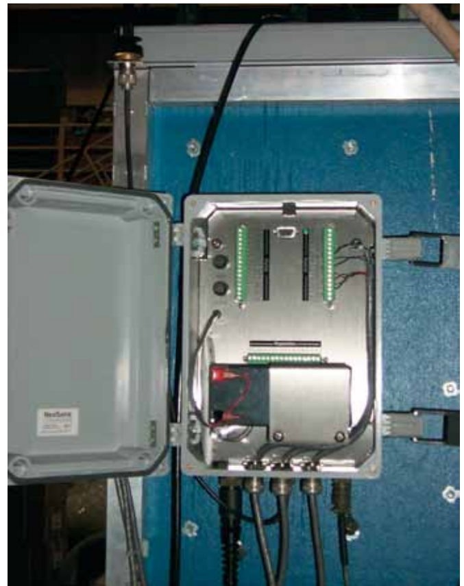
Figure 3.4 Field Communications Enclosure.
