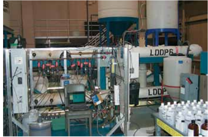
Figure 2.2 DSS Loop No. 6 Sensor Manifold and Instrumentation Rack
