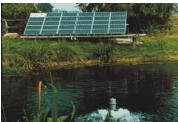
Figure 142: Photovoltaic system for surface pumping
