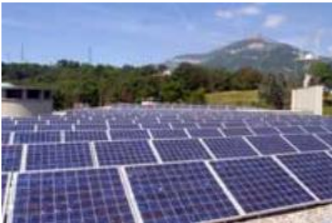
Figure 146: PV power plant in Chambéry (France)
