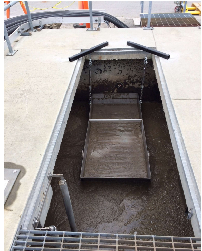
Lamella plate settler installed (without pump)
