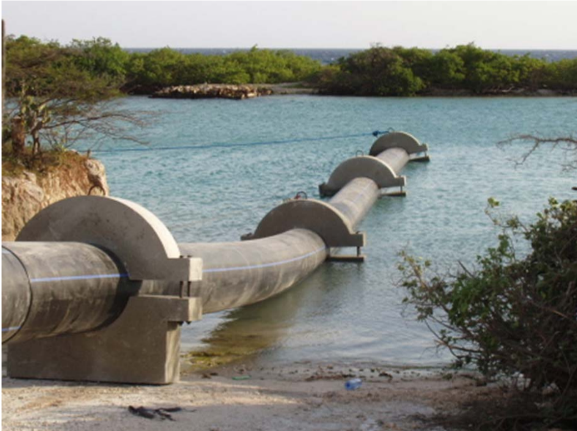
Figure 8 – Concentrate Discharge Pipe
