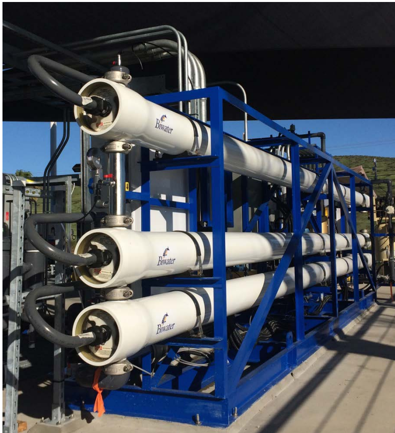
Figure 12. AWP Demonstration Facility primary RO system.
