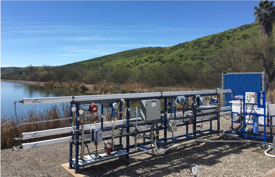
Figure 21. CRRO treatment skid.
