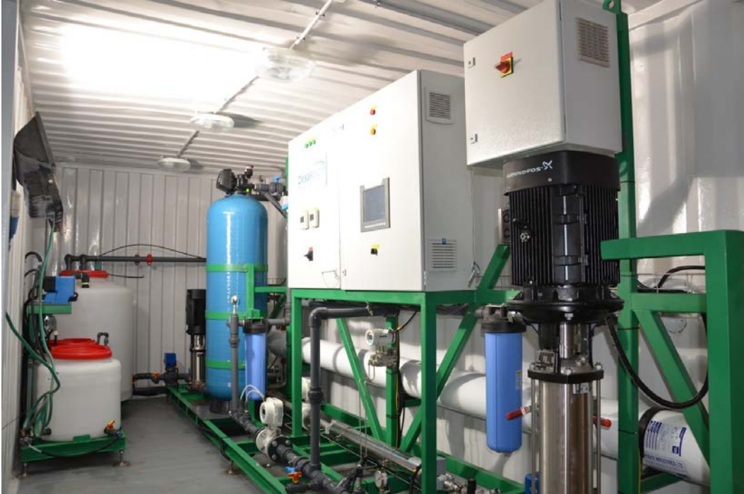
Figure 13. CCD prefabricated container skid by Desalitech.
