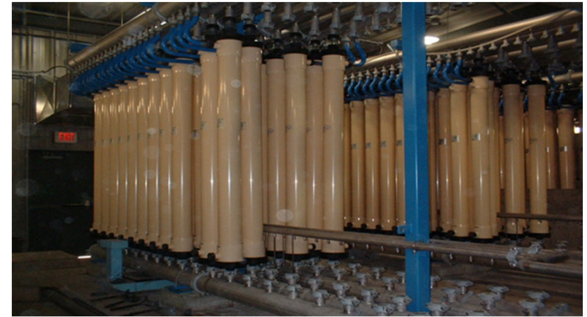
Microfiltration water plant
