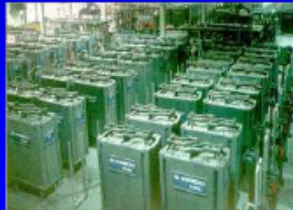
12 MGD Sarasota, FL EDR plant
