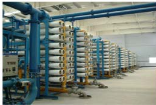
Desalination of seawater plants in Guangdong Jiulong (100,000 t/d)
