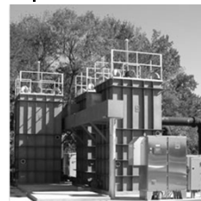
Clayton County, GA NE STP uses five 7' X 7' filters handling up to 15 MGD at 30 gpm/sq ft.
