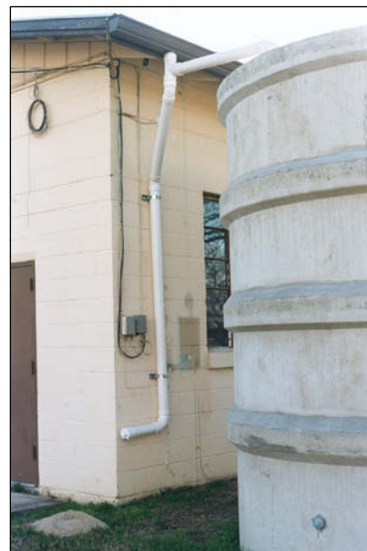
Stacked concrete ring 3,000-gallon tank at the Auld Center, Kerrville, showing first flush diverter and cistern.
