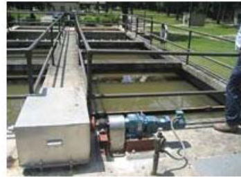
IMG_3622.JPG-Chain and flight at primary clarifier
