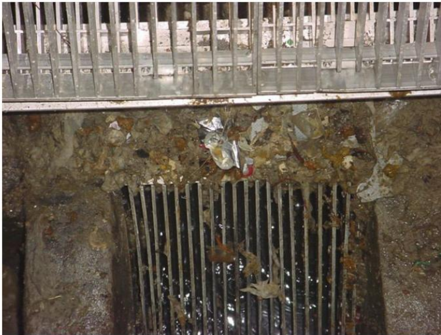
Manually cleaned screens/bar rack – St. George's University Grenada – Daniel & Daniel Engineering Inc
