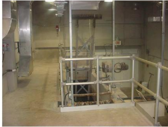
Mechanized cleaning of screens, DOWASCO Wastewater
