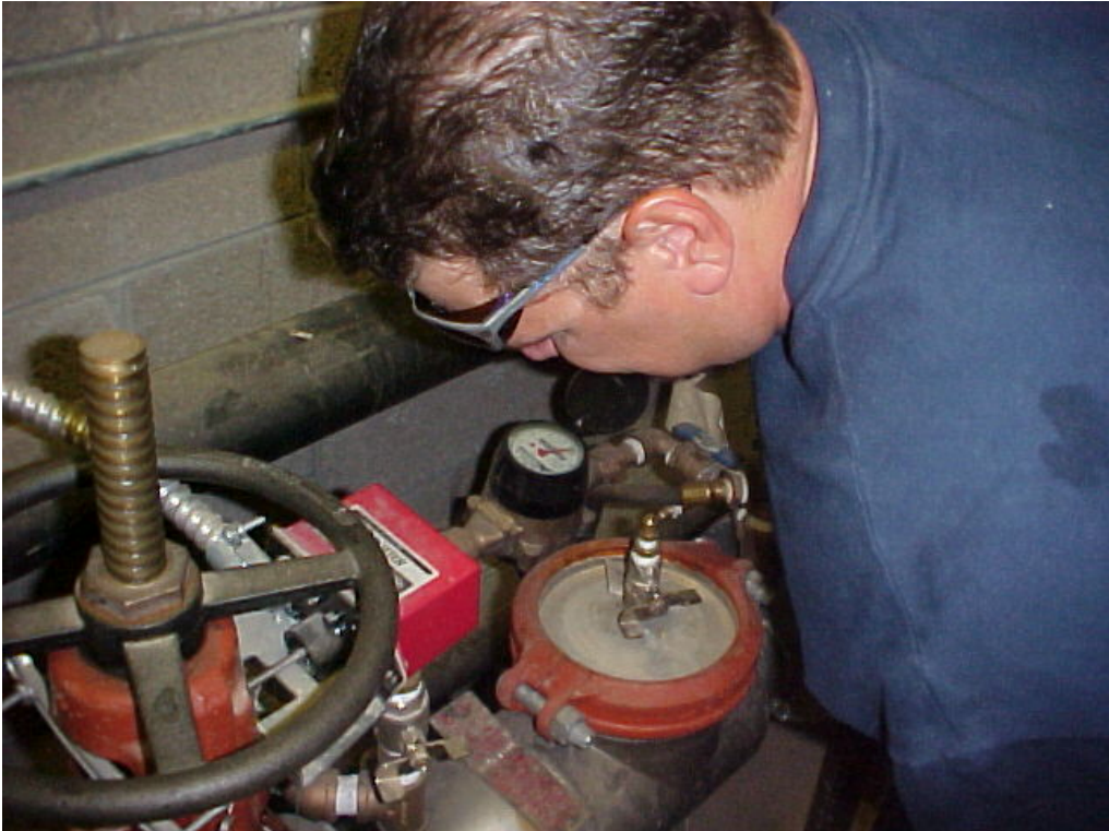
A Certified Tester is testing the integrity of this RP. Notice OS &Y.
