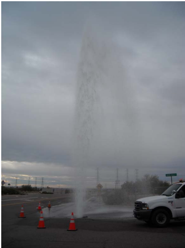
Water main break, perfect time to create a cross-connection. Waterborne
