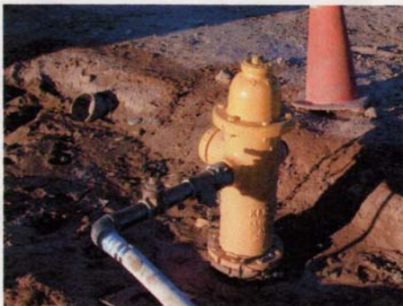
Fitting at hydrant
