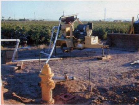
Direct connection from hydrant to pump.
