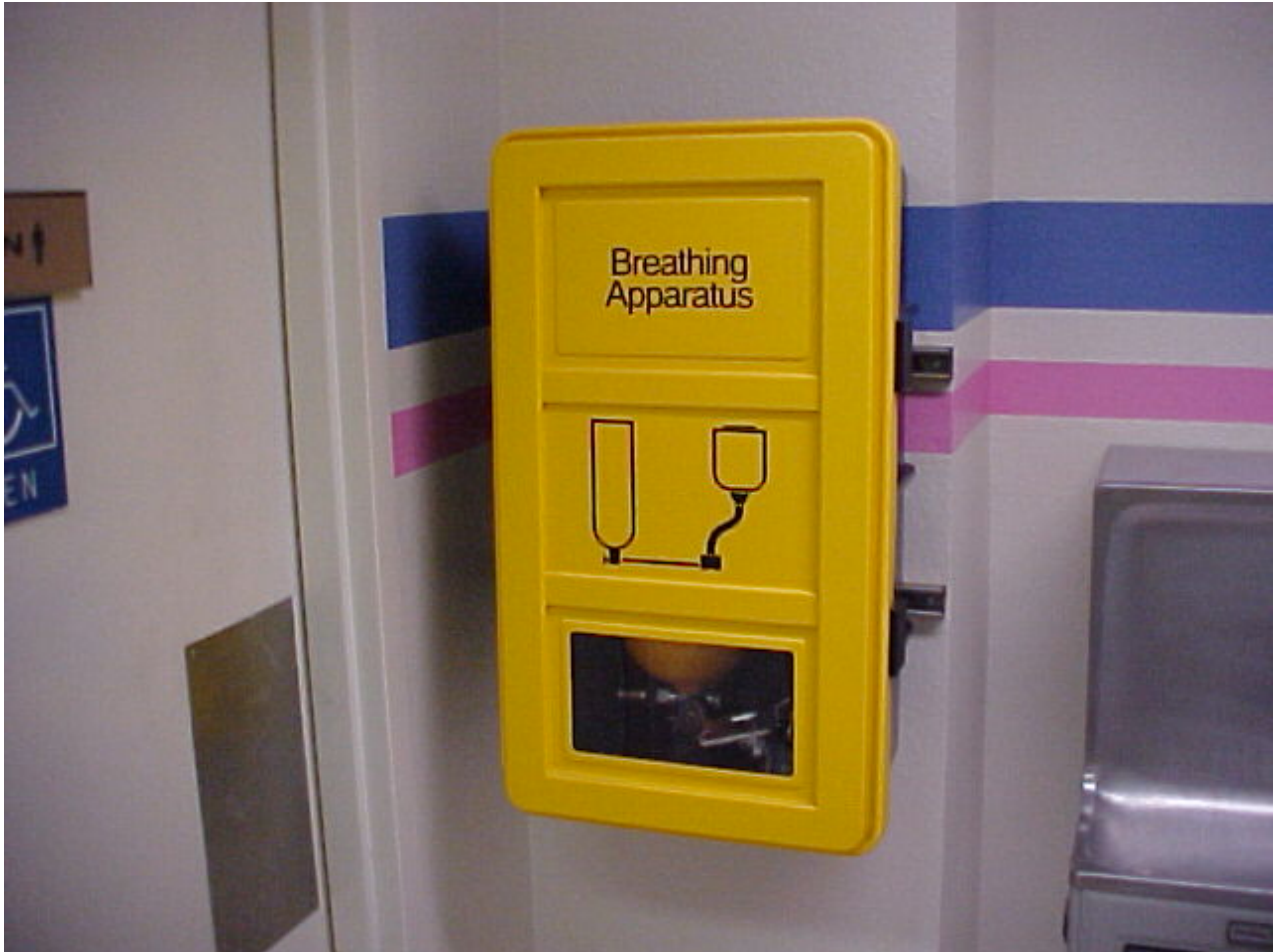
SCBA Storage Box
