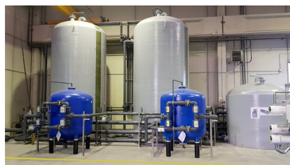
Test bench for large units, Spain
