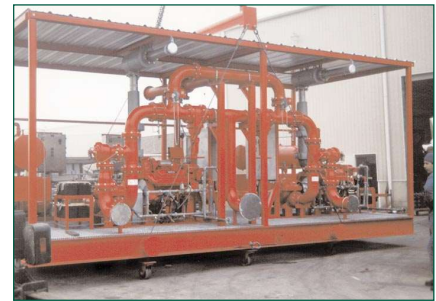
Photo 1. Fire water pump with diesel engine and air start with a nitrogen back-up system
