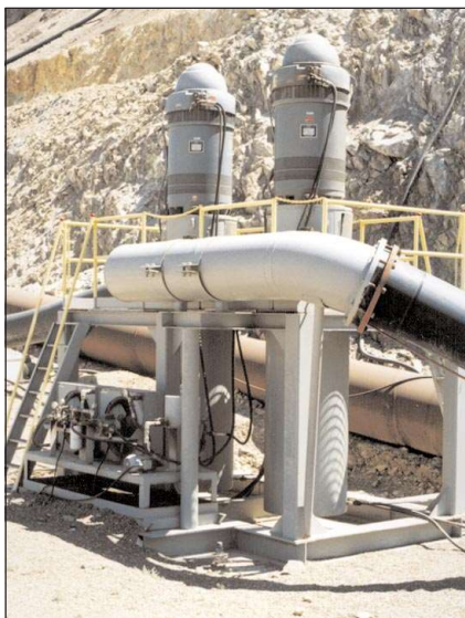
Photo 2. Twin 800 hp, 5000 gpm vertical turbine can boosters with 42" discharge main in background
