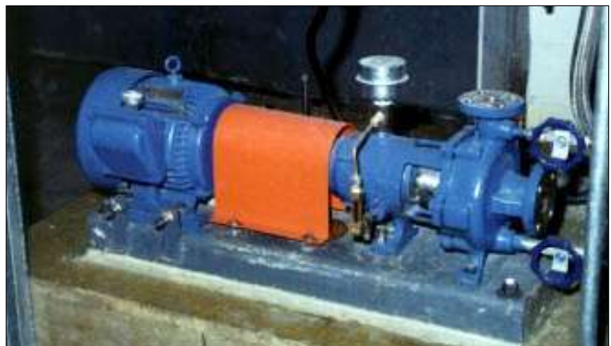
Photo 2. An upgraded second generation pump receives backup as part of the reliability improvement program.
