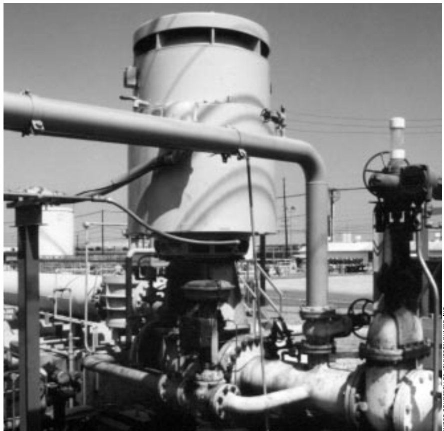
A 500 hp, 1800 rpm product pump operates in a midwest chemical plant.
