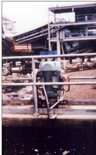
Photo 2. A vertical chopper pump handles bark, wood, rocks and dirt in a pulp mill log yard stormwater runoff sump.
