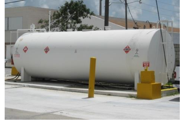
10,000 Gallon Diesel Double-Wall Steel AST
