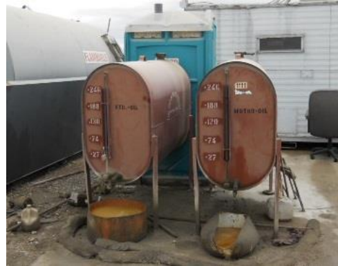
Steel Oil ASTs not in Containment
