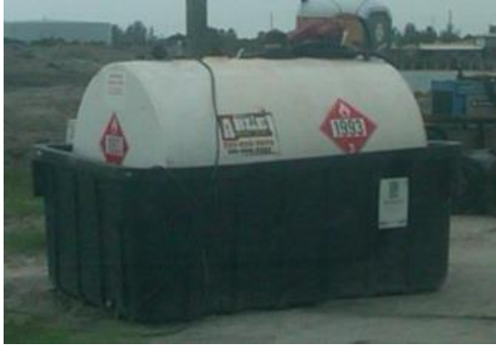
Single-Wall Steel AST in Plastic Containment
