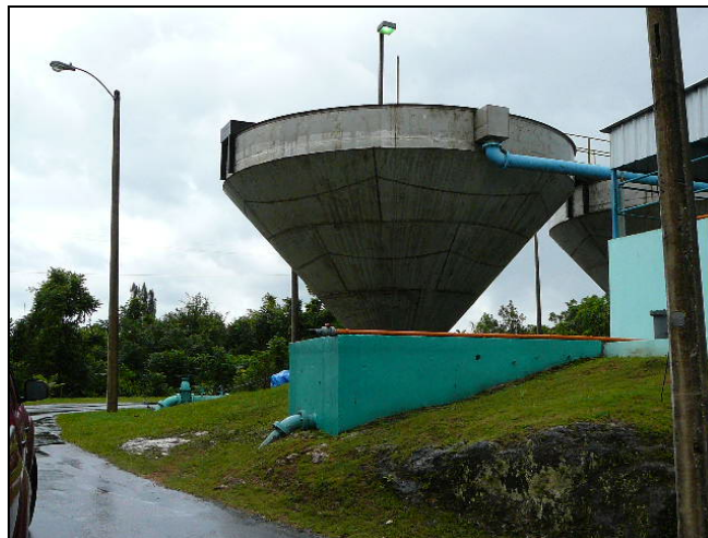
Figure 28: SpiraCone Solids Contact Clarifier Photo by author.
