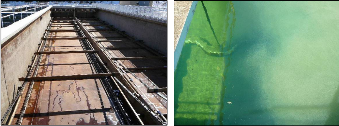
Figure 26: Rectangular clarifier sludge removal system
