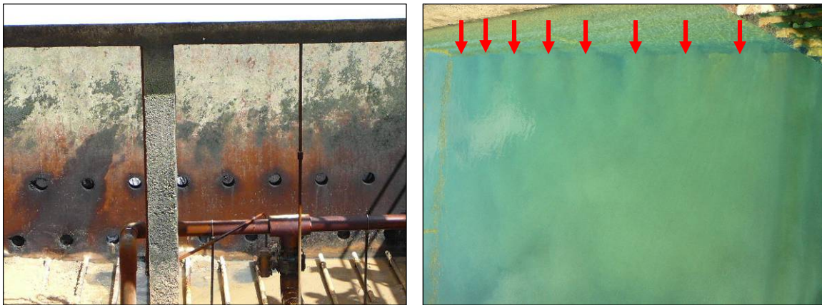
Figure 27: Clarifier w/ perforated inlet baffle wall
