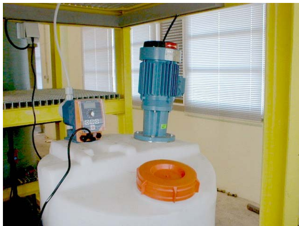
Figure 14 Solenoid pump installed on the dosing tank.
