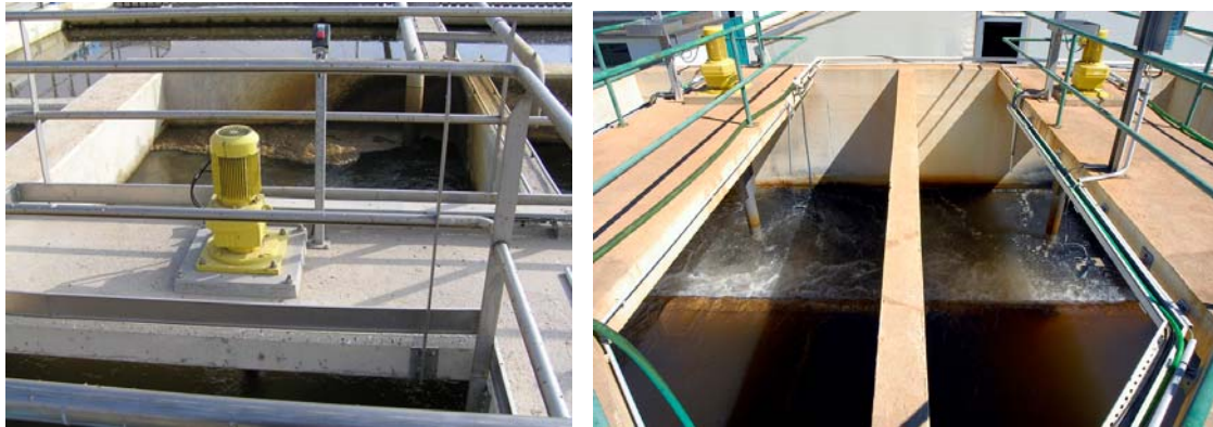
Figure 4 Engines for mixing in coagulation tanks.
