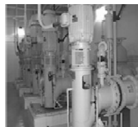
Raw wastewater pumps, Ames, IA
