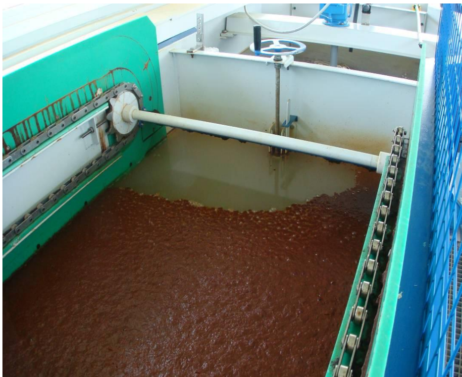
Surface of the floatation tank during normal operation
