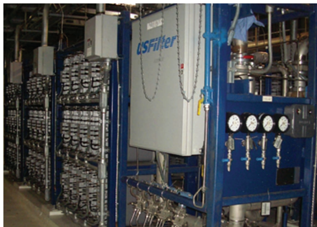
Figure 1 6,750 gpm (1500 m 3 /h) boiler feed water CEDI system (1 of 10 skids). USFilter is now part of Evoqua Water Technologies.
